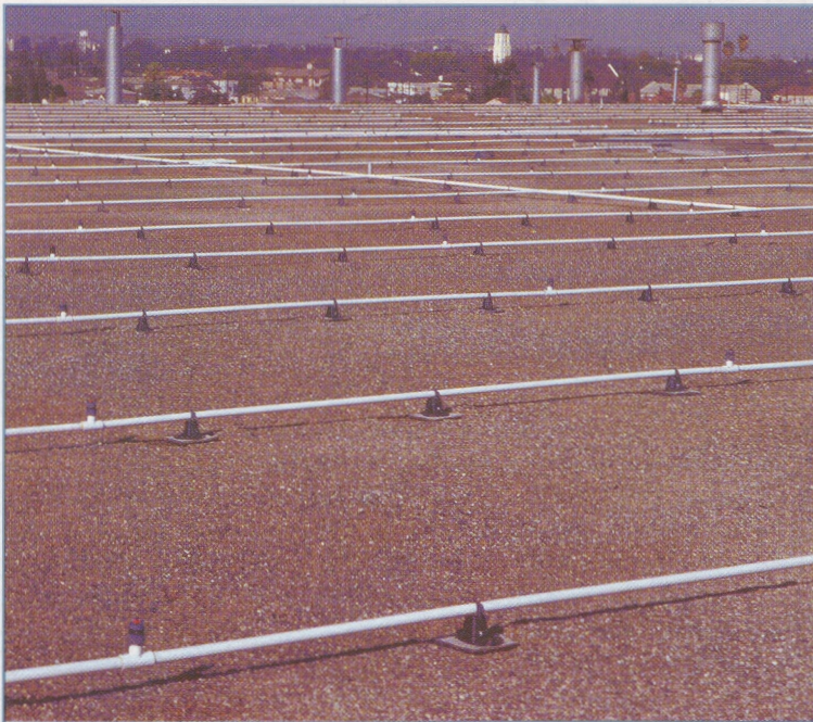
Figure 3: The lightweight piping network is supported every 40 in. by a polymer pipe stand that is sized to allow the pipe to move freely. During each misting cycle, no more water is misted than will evaporate in a short time; hence, standing water is avoided.
