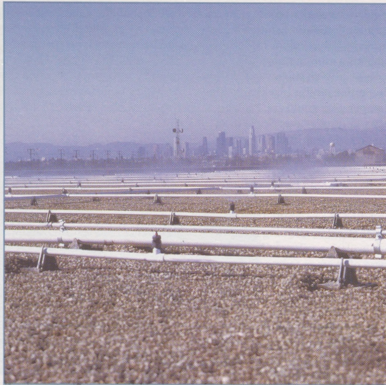
Figure 4: Each sprayhead cools about 100 sq. ft. of roof, leaving wide aisles accessible.
