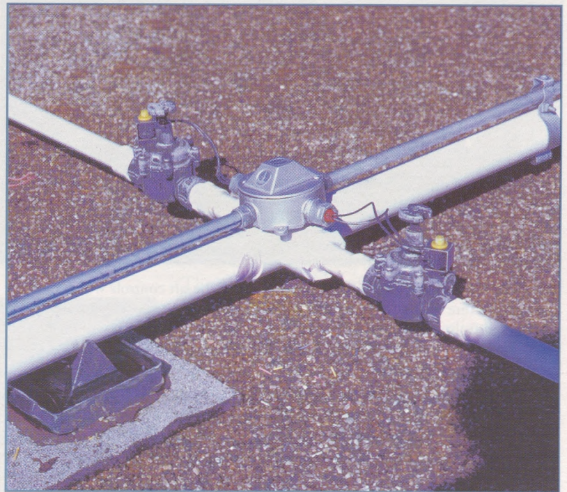
Figure 1: Each low-voltage solenoid valve (24 VAC) controls the supply of water to 50-80 sprayheads, reaching 5,000-8,000 sq. ft. of roof. The 2-in. diameter mainline water supply rests on 6" x 6" plastic supports which are placed at 5' intervals.
