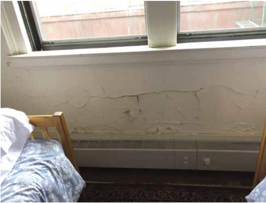
Figure 5. Interior finish damage beneath fenestration was caused by water accumulating between the storm window and the original fenestration unit.
