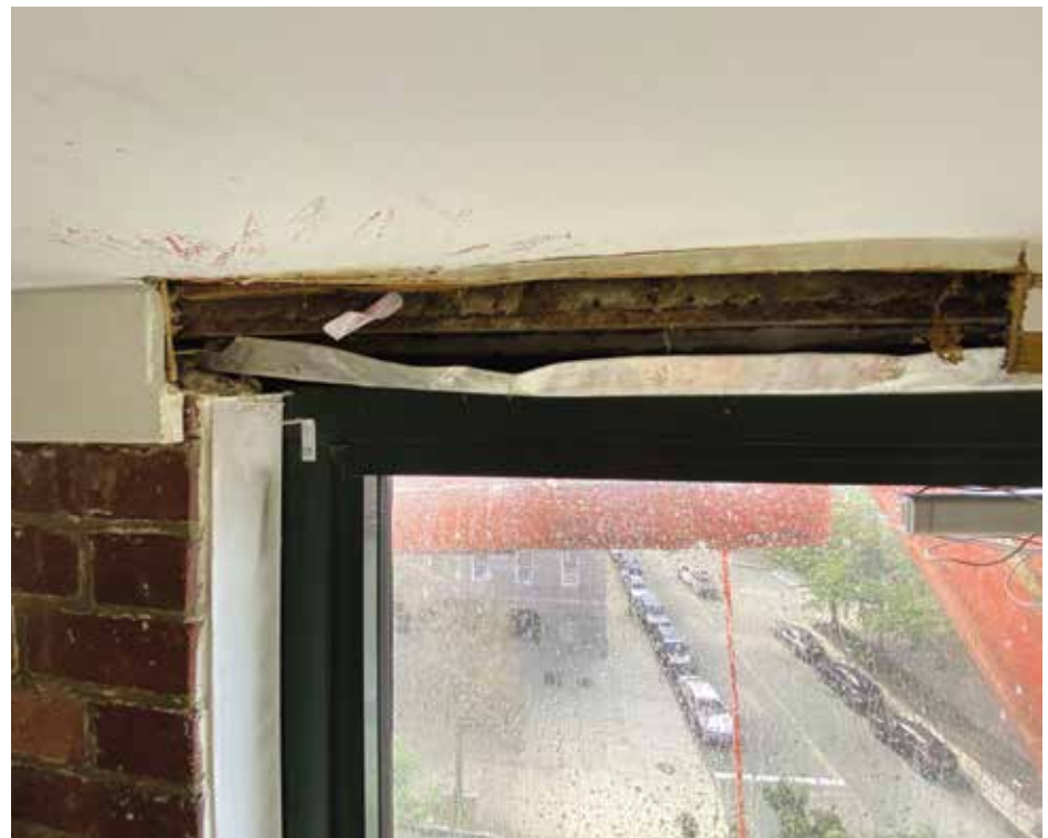
Figure 4. Water leakage at interior appears at window head; however, the leakage path is through exterior masonry wall above.
