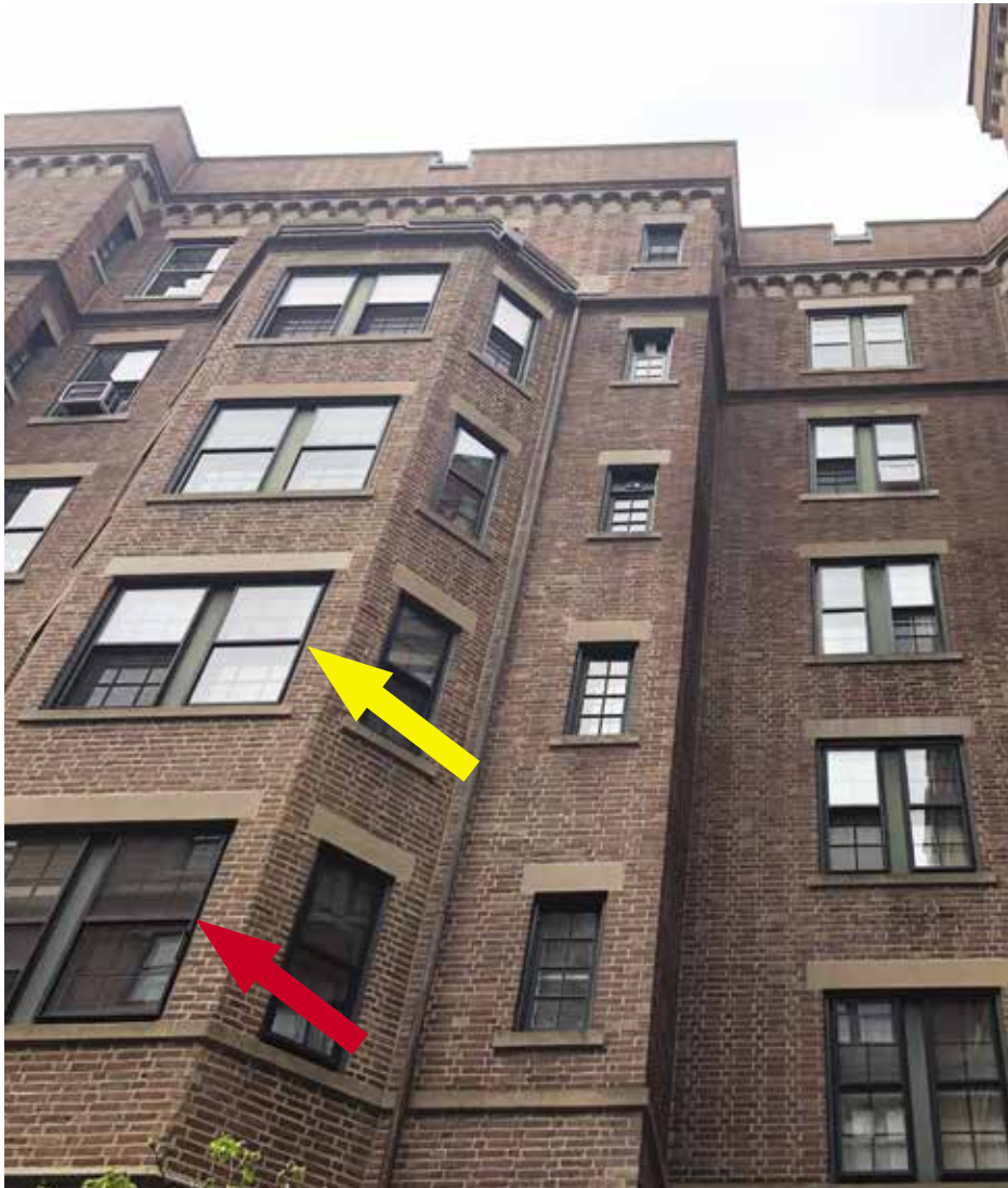
Figure 1. Storm windows installed at localized fenestration of a condominium building. Yellow arrow indicates a location with a storm window; red arrow indicates a location without a storm window.
