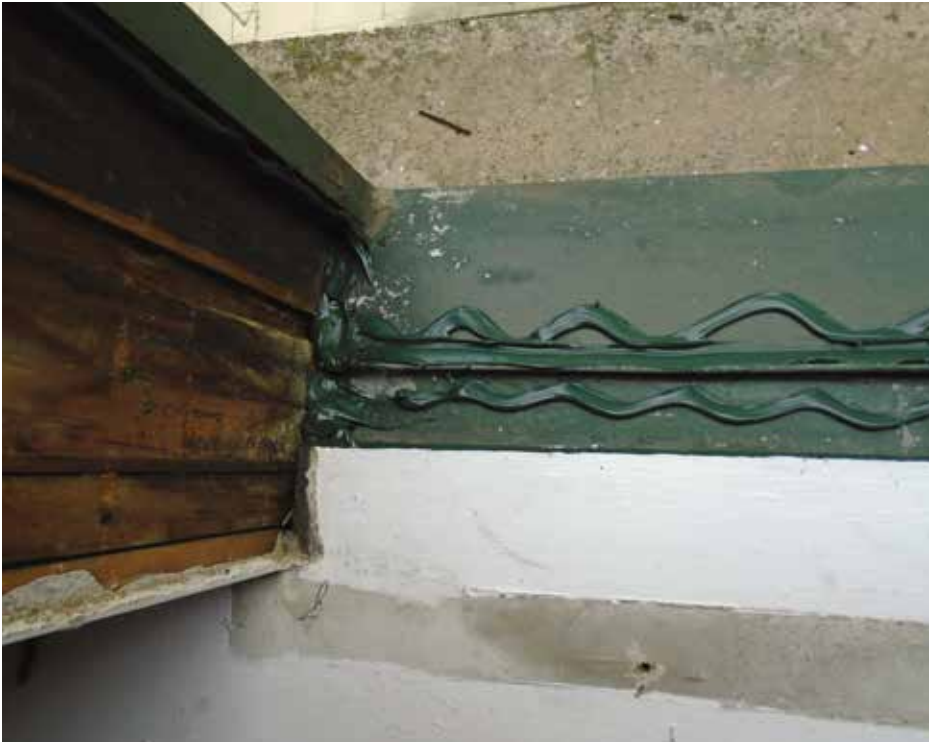
Figure 6. One-off fenestration replacement where the perimeter air/water barrier is limited to sealant.
