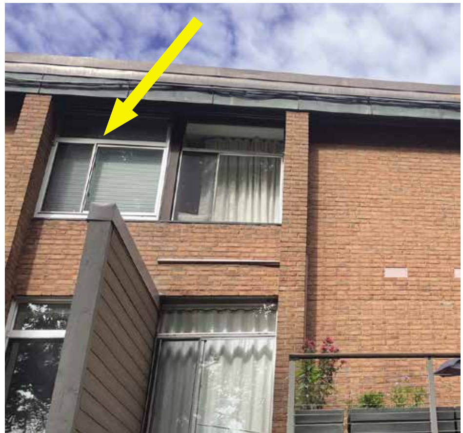
Figure 3. Sight lines at the replacement fenestration (indicated with the arrow) are thicker than existing fenestration profile next to it.
