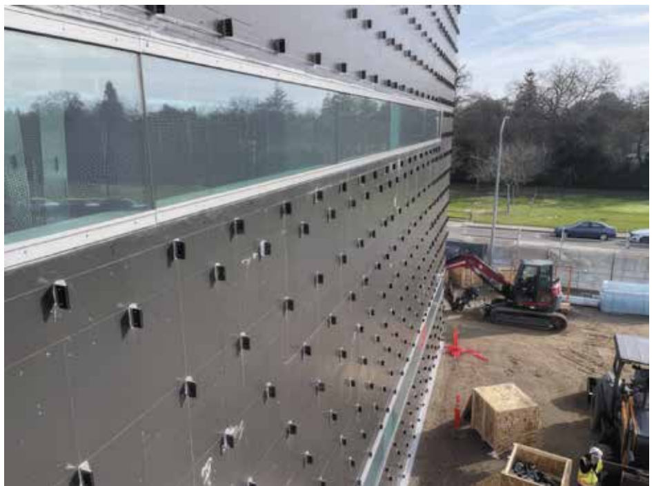
Figure 5. Partial view of an elevation prior to the dry film thickness and chamber depressurization in conjunction with leak detection liquid tests.
