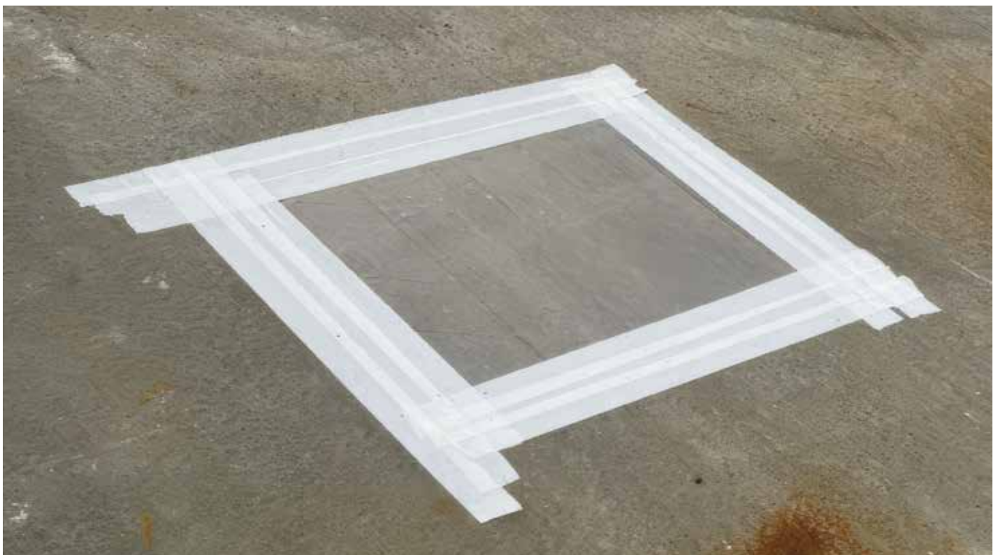
Figure 1. Plastic sheet taped at concrete surface on the roof per ASTM D4263, Standard Test Method for Indicating Moisture in Concrete by the Plastic Sheet Method.
