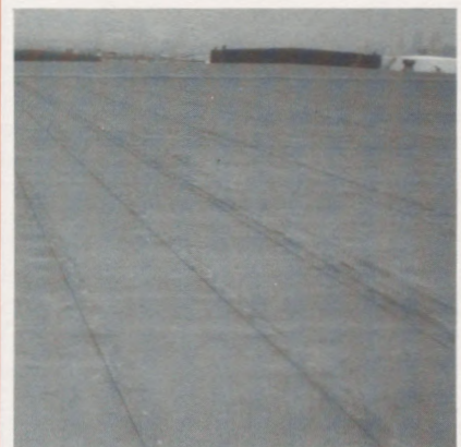
Photo 13 A 1986 installation installed in compliance with ANSI A58.1, the perimeter width measuring 40% of the building height. No corner or perimeter repairs were observed.
