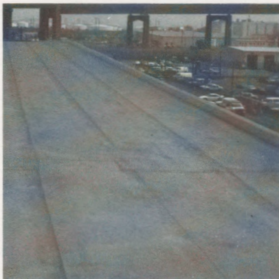
Photo 11 'Early' spot adhered and lap combination system with increased corner and perimeter attachment densities performing well after nine years.
