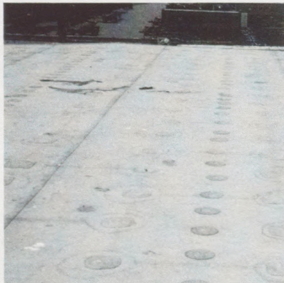
Photo 2 Early installations did not include preliminary insulation attachment. Subsequent attachment and perimeter repairs created an abundance of patches.
