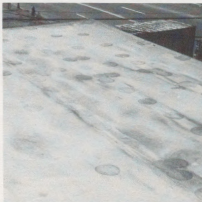
Photo 15 Multiple visits to the same repair area, a prevailing wind corner.
