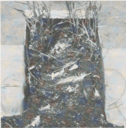
Photo 17 Poor maintenance was a common problem on all roofs in the survey.
