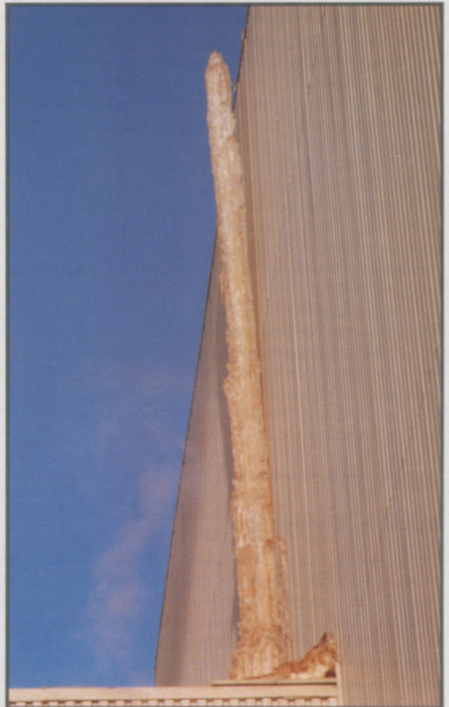
Ice column which is approximately 30 feet high has loosened from the wall and is ready to fall onto the roof below.
