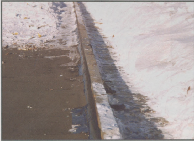
Preparing a joint for membrane flashing installation. Snow is approximately 3' to 4' deep on the right side of the joint.
