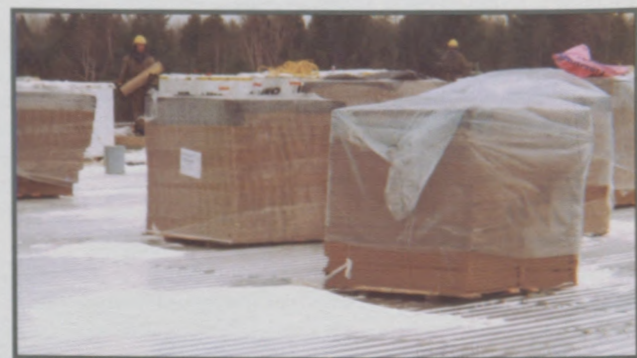
Inadequate storage of insulation and membrane. Rolls should be stored in a warm environment while insulation should be covered with breathable tarpaulins. Factory-applied shrink wraps do not serve this function.
