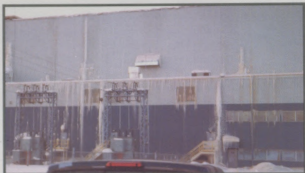
Extent of ice formation on exterior walls caused by lack of perimeter drainage system.
