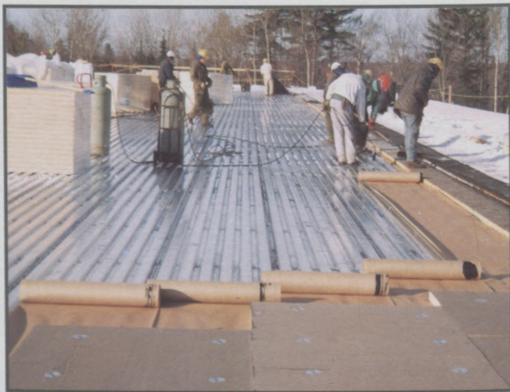
Contractor removing snow from deck flutes and right seal area. Installation of vapor retarder and base insulation is taking place. Temperatures are -15°C at this time of the morning.
