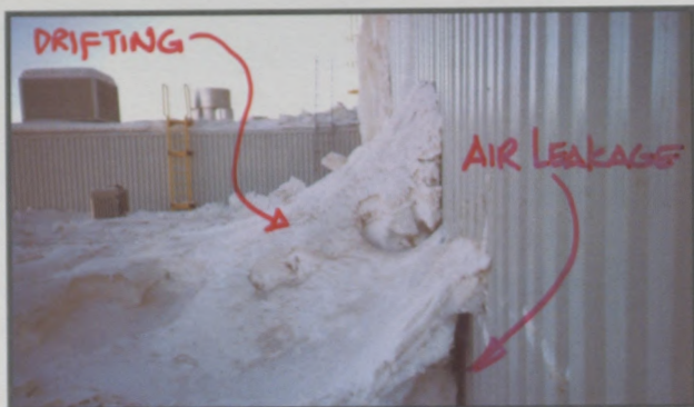
Snow drifting at low roof against wall of higher roof. Drift is approximately four feet at peak. Air leakage has also created a cavity at the base of the wall. During snow melt, water can accumulate in this area and enter behind improperly-sealed flashings.
