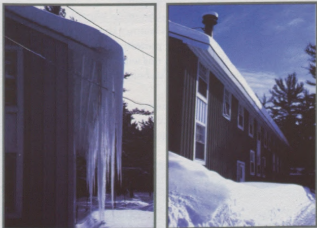
Figure 1: Two identically-constructed roofs photographed at the same time. The building on the right, with no icings, was unheated.
