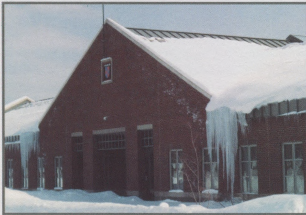
Figure 3: Minor icings occurred along the eaves of this roof and problematic icings developed at the base of valleys.
