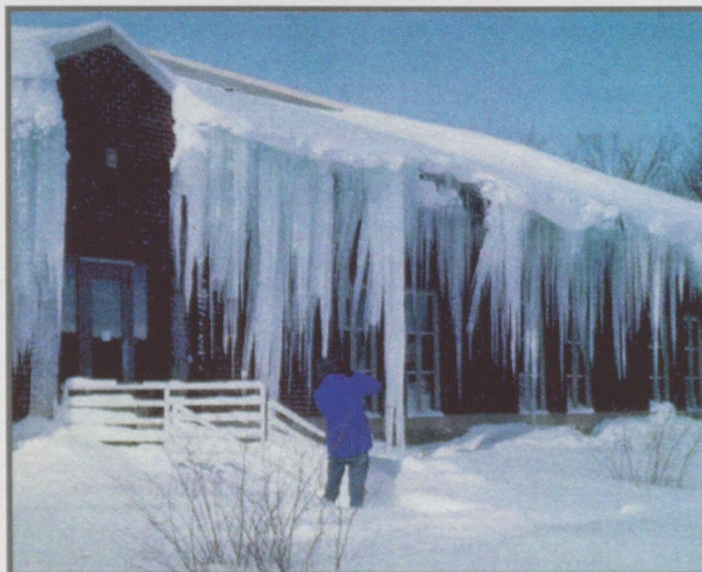
Figure 4: Severe, problematic icings developed all along the eaves of this dining facility.
