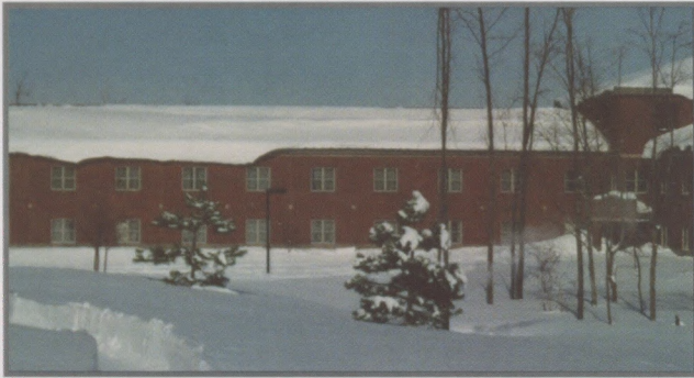
Figure 2: Some creep of snow and cornicing is evident, but no icings occurred on this roof.
