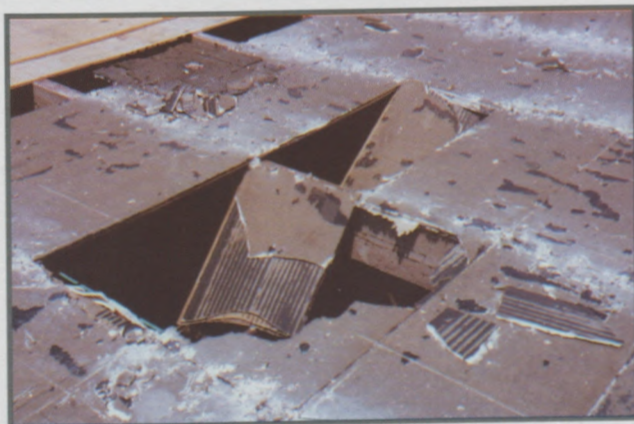
After the roof was removed, the sheetrock deck was found to be in worse shape than originally anticipated.
