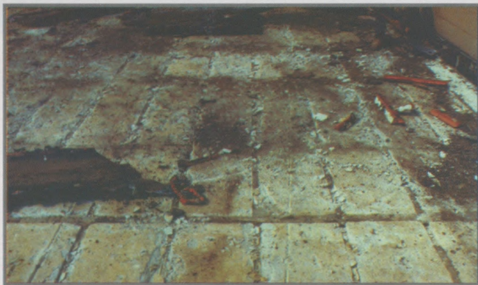
Figure 2: LAACCRP roof panels as viewed upon the removal of the existing roofing. Note the surface deterioration.
