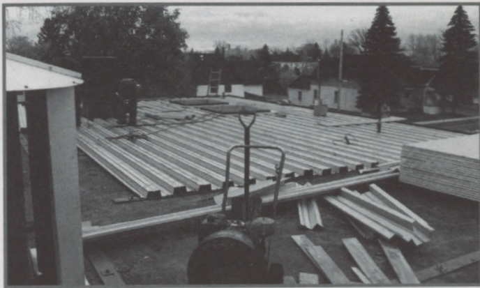
Figure 4: The LAACCRP roof deck was found to be unable to resist the snow loading. A new structural system is being installed, consisting of 25 mm deep x 25mm wide steel plates welded to the supporting steel structure below accessed by drilling cores through the LAACCRP. New 75mm deep corrugated steel decking is being fusion welded to the plates and will span the required 2900 mm, which is the span between the new plates. Although the LAACCRP is not being removed, it will no longer be required to resist any loading other than its own weight.
