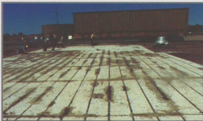
Figure 3: LAACCRP as viewed after the grouting of the surface deterioration. This section is now ready for priming and new roofing assembly.
