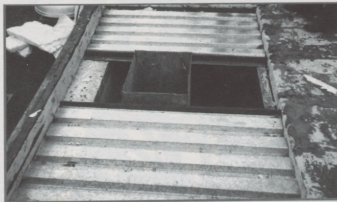
Figure 5: LAACCRP roof panels found to be severely deteriorated have been removed and replaced with new 38 mm deep corrugated steel decking. The new steel deck is fusion welded to the existing steel beams and anchored to the exterior masonry block wall.
