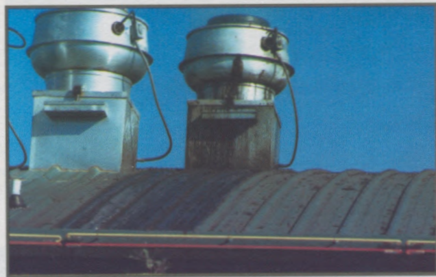
Grease discharged on surface of metal panel roof system.
