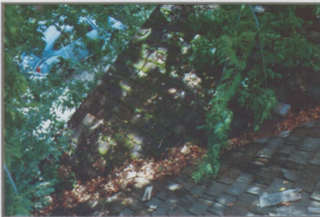
Moss growth on wood shingle roof covering.
