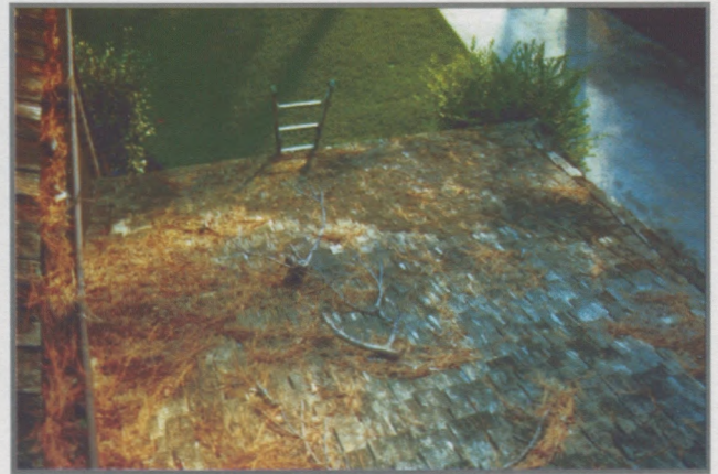
Pine needle accumulation on wood shingle roof covering.
