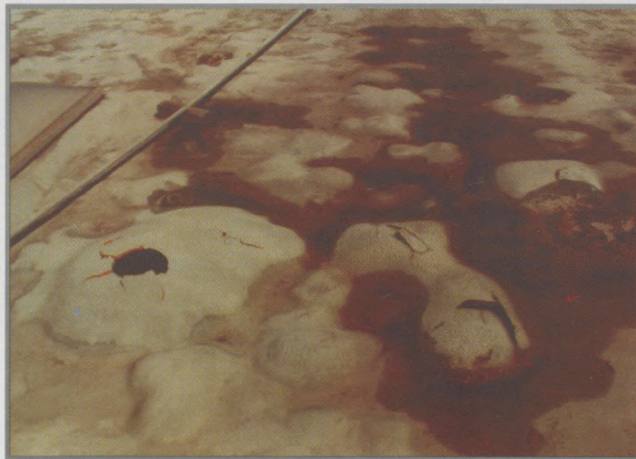
Blisters in spray-applied polyurethane foam roof system.
