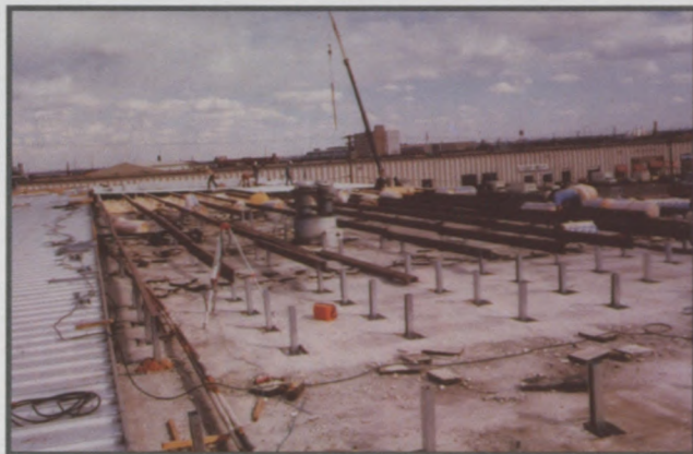
Figure 6: Retrofit metal roofs have, on occasion, induced drying of old materials left in place. The attributes of plenum ventilation are largely responsible. (Photo courtesy Rob Haddock.)
