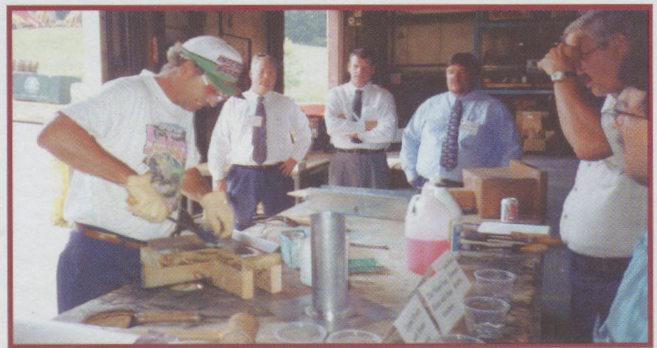
Ed Wright of Citiroof Corporation demonstrates techniques and provides insights for soldering various types of metal at a recent Region I meeting of RCI.
