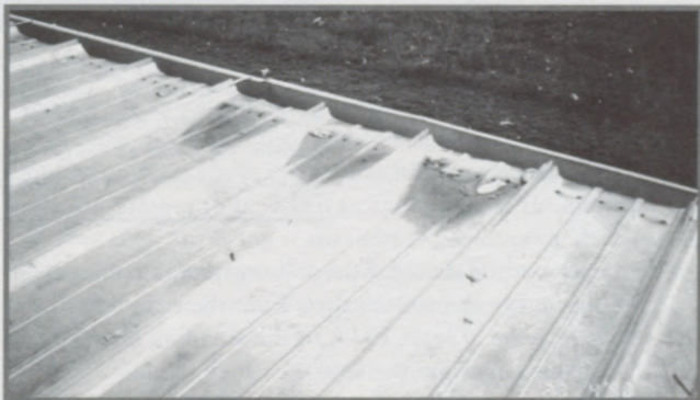
Shown here is a failure to provide required structural support at the eaves. As a result, "cupped" panels hold water, there is damage to the Galvalume coating on the panels, and water is forced back into the building at the wall and eave lines.
