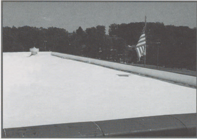
A completed job shows the aesthetic value and high reflectivity of white roof coatings. RCMA and Oak Ridge National Laboratories are currently researching the effect of reflective roof coatings on the reduction of heat flow through the roofing system and aging of roofing membranes.
