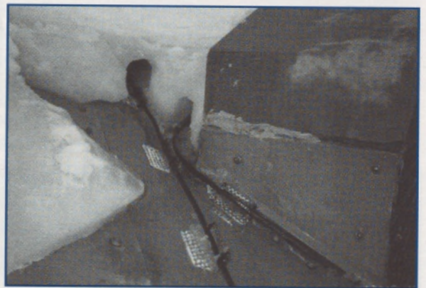
Figure 8. Heaters provide melt paths through snow and ice for meltwater to drain off the roof. Some ice was removed to expose these paths for this photo.
