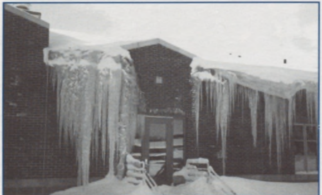
Figure 1. Severe, problematic icings and ice dams along eaves of a dining facility at Fort Drum in upstate New York.
