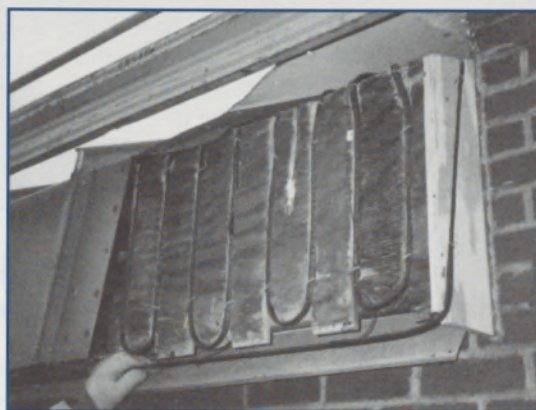
Figure 11. Heater laid in channels routed in the plywood sheathing behind the fascia metal.
