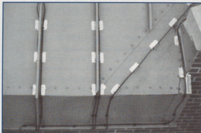
Figure 6. Typical attachment of nylon mounts to fascia with epoxy. Angle clips on the roof itself are attached with neutral-curing silicone. Note horizontal heater all along drip edge.
