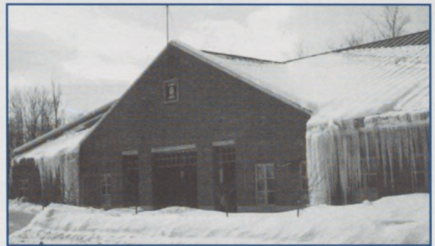
Figure 2. Large ice dams and icicles form where the gable parapet ends at the bottom of valleys.
