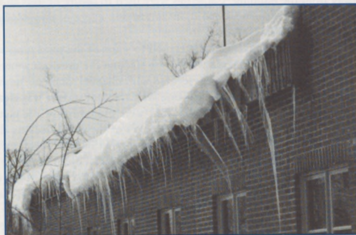
Figure 15. Icings forming on a creeping, overhanging mass of snow and ice, bypass the heated fascia on this building. Note exposed heaters at near end of fascia.
