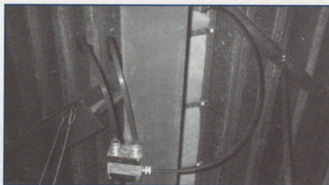
Figure 5. System with high output heater installed below the metal roof in a valley.
