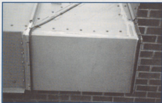
Figure 13. False closed-top fascia installed over heater shown in Figure 12. Note heated vertical baffles (water diverters) at each end.
