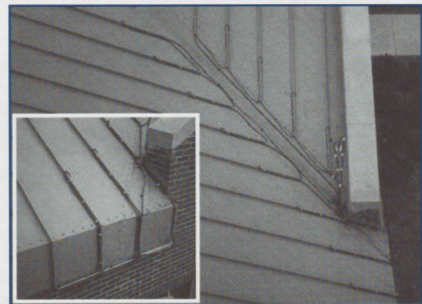
Figure 4. System with multiple heater runs in the valley, behind the parapet and on several standing seams. Inset shows heater runs at its fascia and drip edge.
