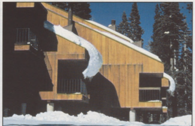
An interesting example of snow sticking to a metal roof. Camellian Bay (Lake Tahoe), CA, February 1985. © Ian Mackinlay
