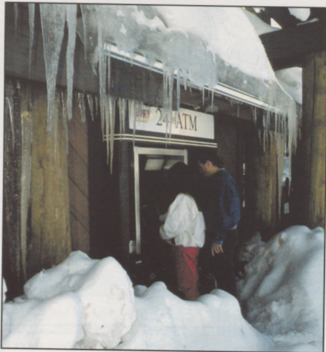
The danger of ice dams on sloping roofs. An accident waiting to happen. King's Beach (Lake Tahoe), CA, January 1993 © Rob Mackinlay
