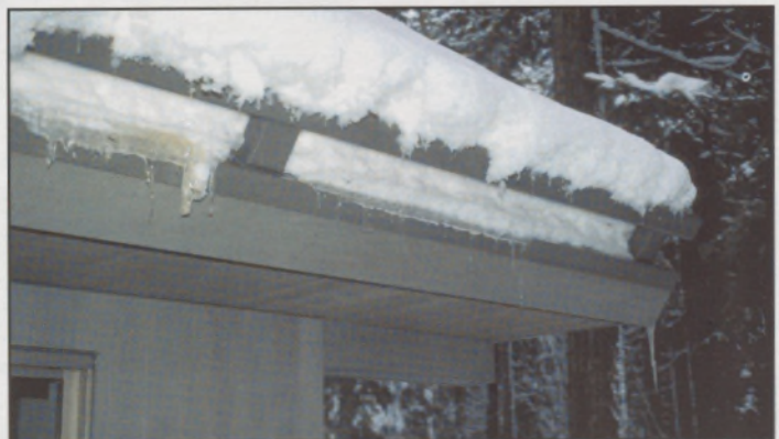
A heated gutter up-roof of a snow arrester. Incline, NV. © Ian Mackinlay
