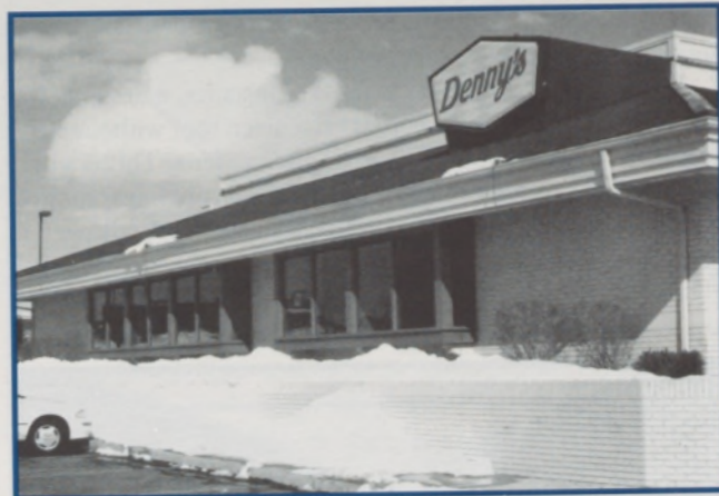
Figure 6: Snowshed here poses a serious threat to both pedestrian and vehicular traffic, as a walkway and parking area are located directly beneath the eave. Note the loose wires hanging from the eave line where light fixtures used to be. Snowguards would have prevented this. (Colorado Springs)
