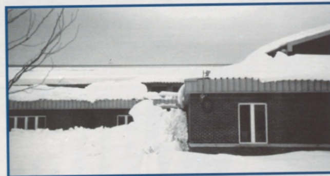
Figure 9: Snow can exert incredible forces on building walls, and lead to collapse if not designed to sustain such force.
