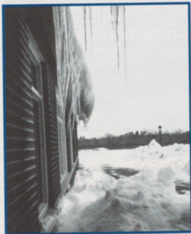
Figure 8: The migration of snow and ice from this roof threatens the glass below the eave. Snow which has previously evacuated the roof is now piled below such that its thaw and drainage from the roof are now directed toward the building wall and foundation. When the pile gets deeper, the runoff will be directed right into the windows
