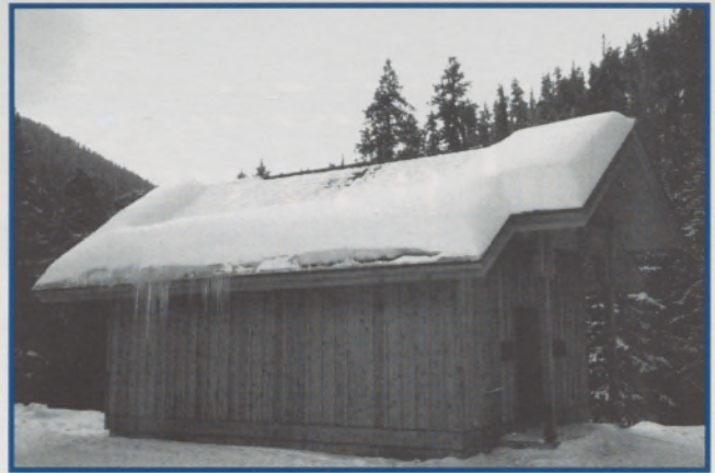
Figure 2: This restroom facility on a Keystone, Colorado ski slope typifies the eave icing effect with its cold overhangs and heated space upslope. Notice that where the heated space has melted the snowbank, the meltwater has run down to a cold eave, forming an ice-dam, which then functions as an unintentional snow guard. At the right, where the roof temperature is consistent from eave-to-ridge, no eave icing.
