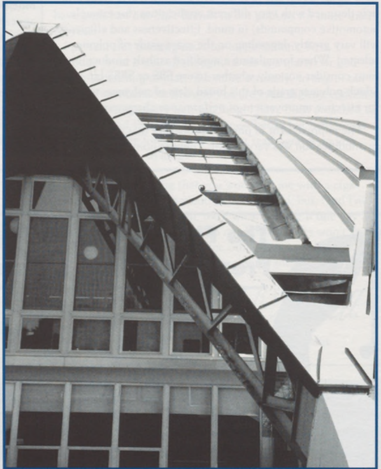
This is a retrofit of a school library. The original hand-made copper roof had a radius of approximately 103 feet. 3-3/4"-deep hat sections were spaced at five feet on center over the old roof with fiberglass blanket insulation and a Butler MR-24 Roof System in a green patina (weathered copper-color) Kynar paint finish.
