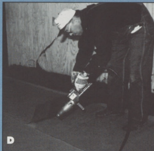
Figure D—End laps make a T-joint in the cutout area, where extra adhesive is then placed.
