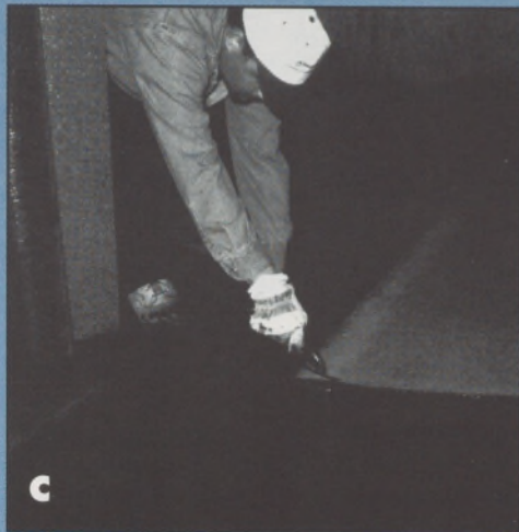
Figure C—The roofing mechanic cuts 45-degree dog ears at the corners of the underlying sheet.
