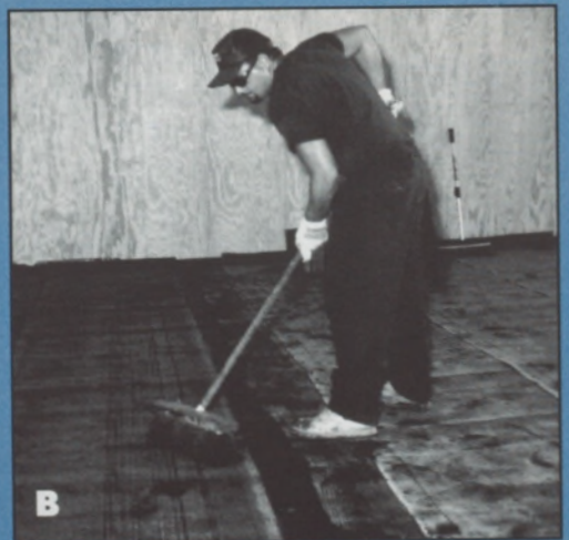
Figure B (right)—Pressure is applied with a broom to embed the membrane firmly in the adhesive.
