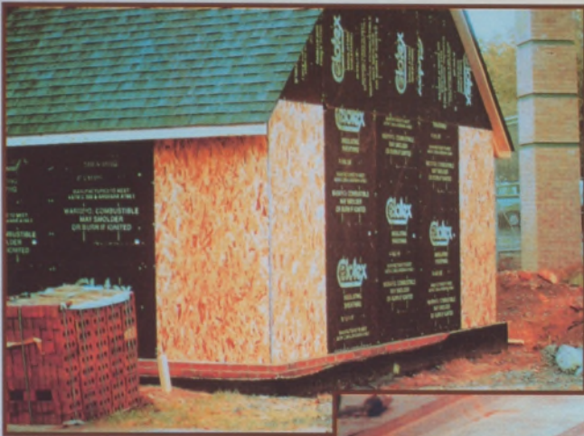
FIGURE 5. PLYWOOD IS USED AT CORNERS OF FRAMED WOOD WALLS, SUBSTITUTING FOR ORDINARY SHEATHING USED ELSEWHERE. THE PLYWOOD IMPARTS HORIZONTAL SHEAR RESISTANCE TO THE FRAMING.
