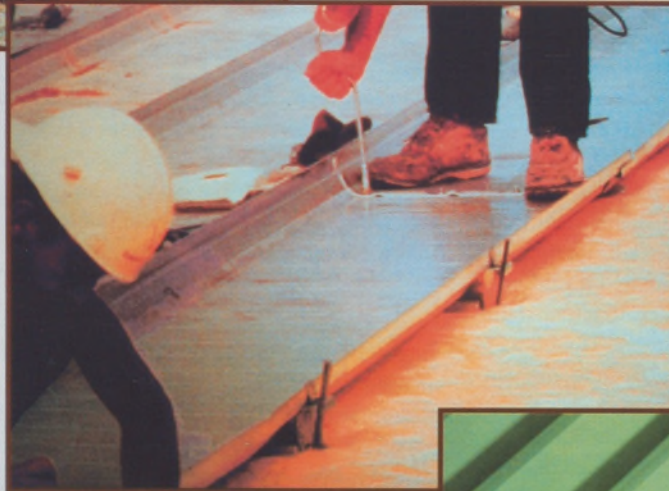
FIGURE 6. STRUCTURAL METAL ROOFS ARE CARRIED ON A SYSTEM OF CONCEALED CLIPS, ALLOWING LONGITUDINAL MOVEMENT OF THE PANS. BEING, THEREFORE, SEPARATED FROM THE STRUCTURE, THE ASSEMBLY IS INCAPABLE OF SERVING AS A SHEAR DIAPHRAGM.
