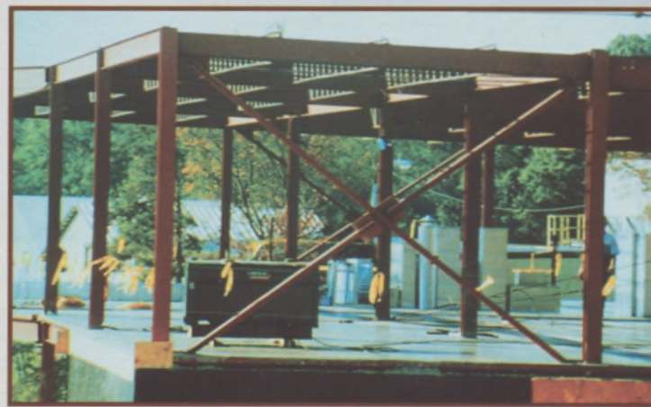
FIGURE 4. A STRUCTURAL SYSTEM HAVING ONLY VERTICAL AND HORIZONTAL MEMBERS MUST BE STIFFENED AGAINST HORIZONTAL LOADS. SHOWN HERE IS ORDINARY DIAGONAL BRACING USING STEEL SECTIONS.
