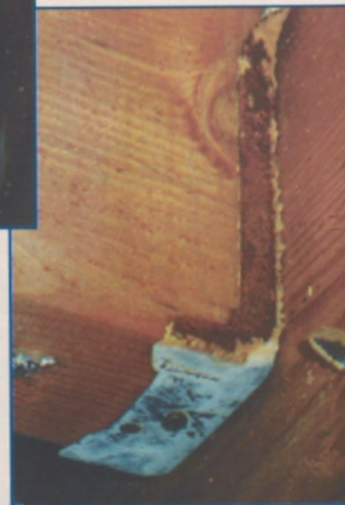
SURFACE RUST ON SIDE OF SUB-PURLIN HANGERS.
