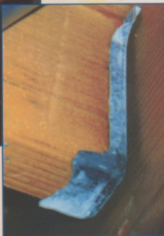
CLEAN SUB-PURLIN HANGER WITH WHITE POWDER BEGINNING TO FORM
