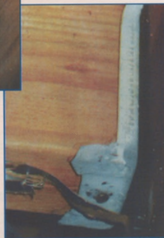
WHITE POWDER COVERING ENTIRE SUB-PURLIN HANGER
