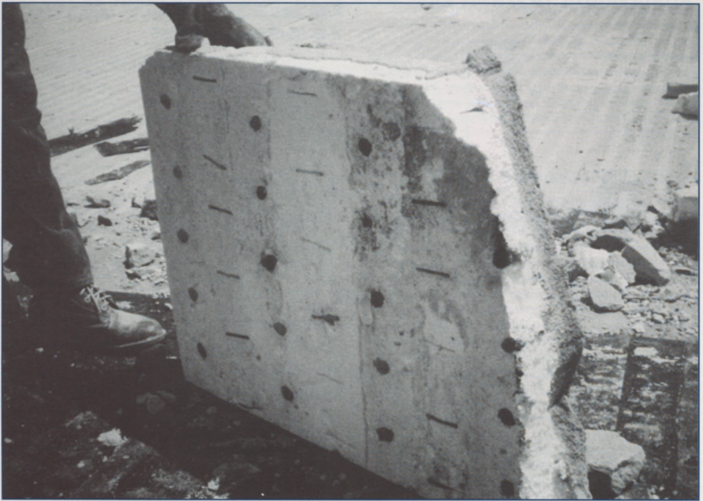
Aggregate-based material with inadequate bond at slurry coat.
