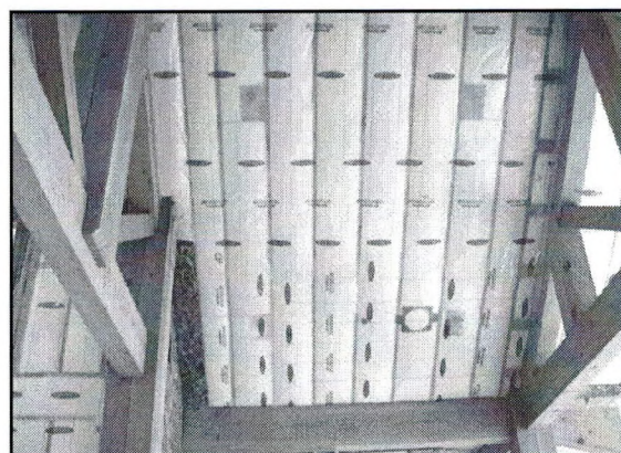
Figure 13 – Airtight unvented cathedral-roof/ceiling assembly with air-impermeable insulation in an extreme cold and dry climate.
