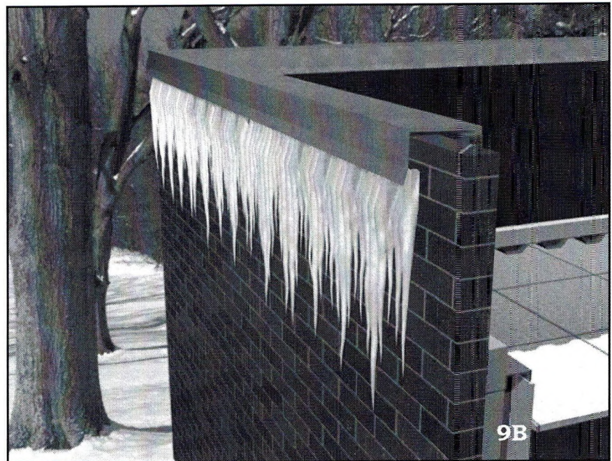
Figures 9A and 9B – Air exfiltration through suspended acoustical ceiling that penetrates the building envelope at the roof parapet and wall interface (9A) causes airborne moisture to deposit at the roof-wall intersection, creating icicle formation during the winter season (9B).
