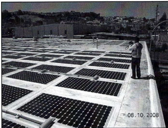
Figure 2 – PV arrays can inadvertently direct foot traffic close to unprotected roof edges.
