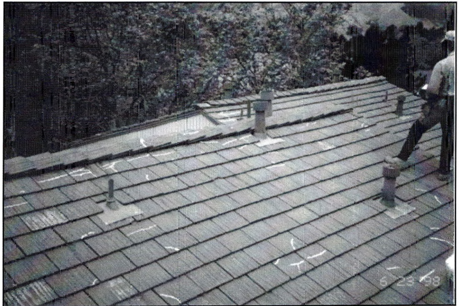
Figure 3 – Seals over fractures in an older fiber-cement roof product.
