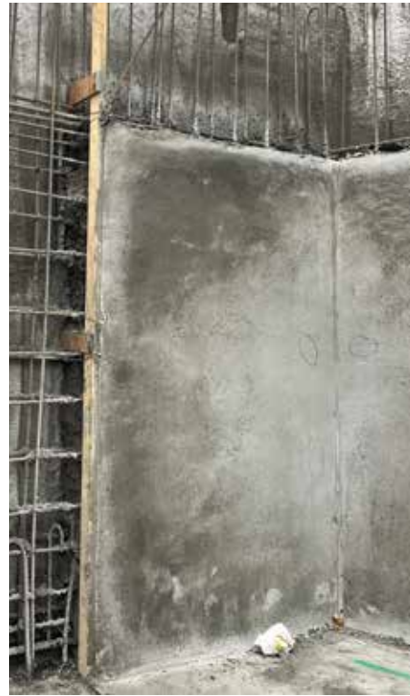
Figure 4. Shotcrete installation on sheet membrane and overspray is approximately 2 ft (0.6 m) beyond construction joints.
