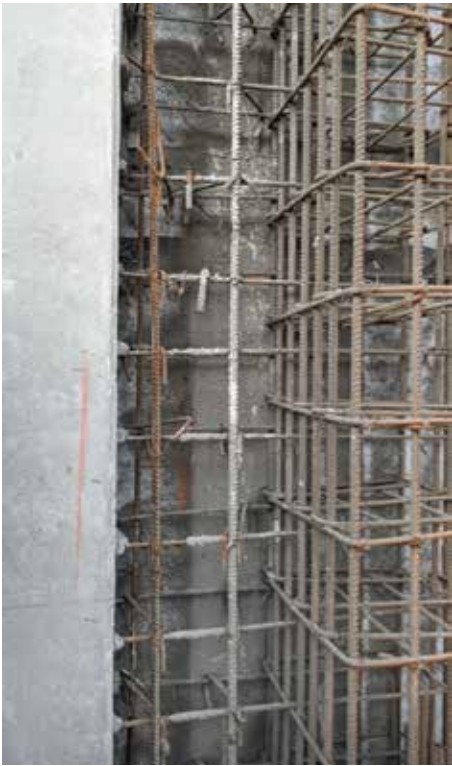
Figure 3. Shotcrete overspray on sheet membrane after form work was removed. No additional overspray removals were expected.
