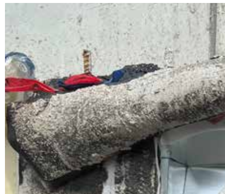
Figure 18. Concrete splatter is found on overlap joint above the concrete pour.
