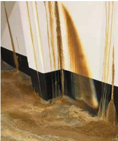
Figure 5. Water infiltration through foundation wall at column location.
