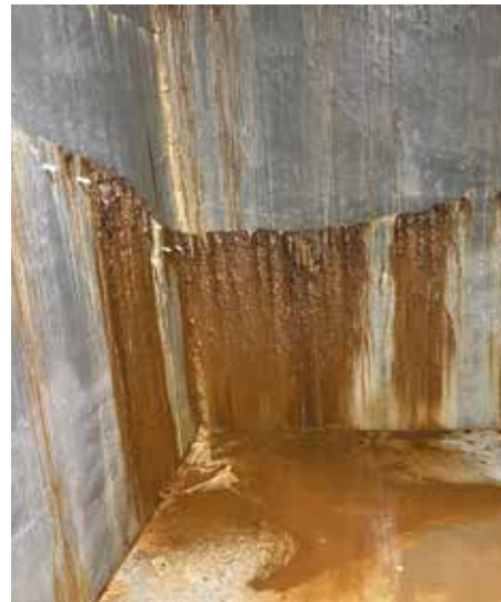
Figure 6. Water infiltration through foundation wall cracks at corner.
