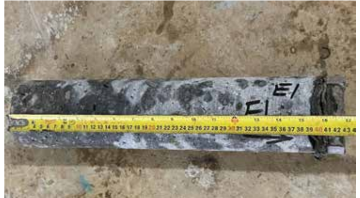
Figure 12. Extracted core of foundation wall waterproofing where the membrane was not adhered due to shotcrete overspray.
