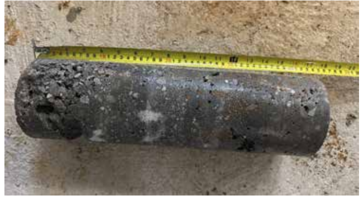
Figure 8. Extracted core from foundation wall showing unconsolidated concrete.
