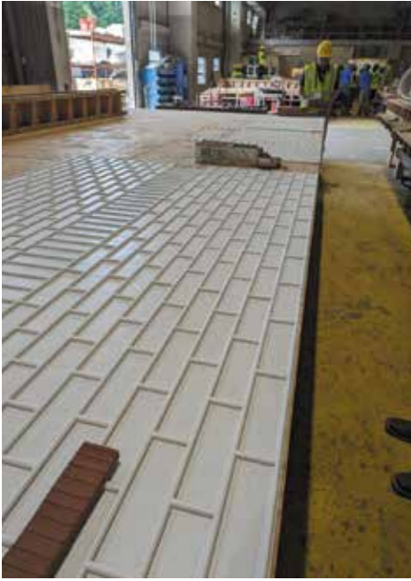
Figure 2a. Thin bricks are placed in form liners like the one pictured here, before concrete is placed. This sets the coursing pattern for the finished wall.
