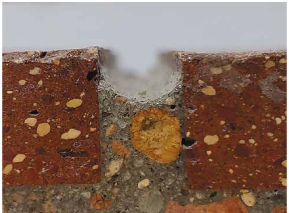
Figure 3. Traditional brick facades use 750 to 2,500 psi (5.2 to 17.2 MPa) mortar between bricks. In a precast concrete thin brick wall assembly, the space between the bricks uses 5,000 psi (34.5 MPa) concrete, which is stronger and more durable.
