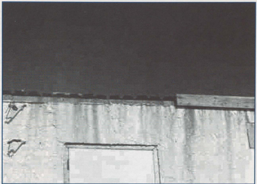
Figure 7: Roof and insulation blown off after edge system failed during Hurricane Hugo (W.P. Hickman Company photo).
