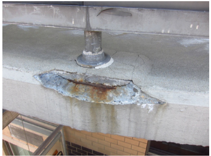
FIGURE 9. View of guardrail post base and balcony edge distress. Photo by author.
