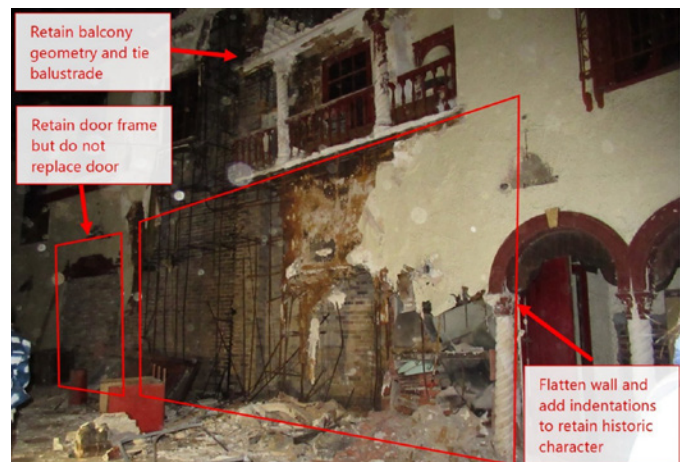
FIGURE 6. Interior view of the theater space showing the plaster conditions of the auditorium prior to repairs, highlighting repair scope.
