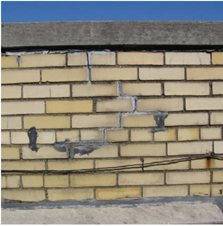
FIGURE 10. View of gap at coping stone, resulting in parapet masonry distress below. Photo by author.
