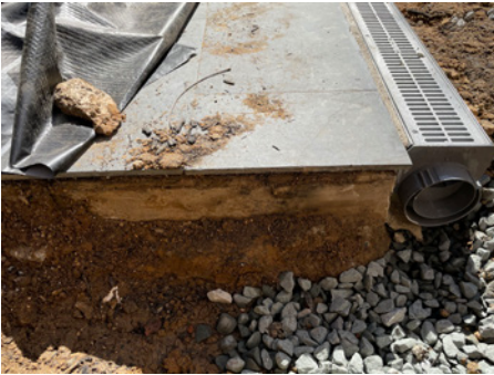
FIGURE 12. The foundation waterproofing did not extend to the top of the foundation walls.
