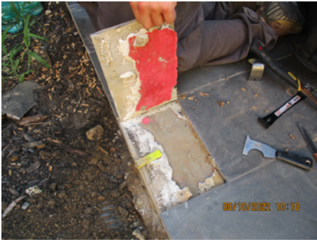
FIGURE 11. The patio waterproofing failed and was not tied into the wall or foundation.
