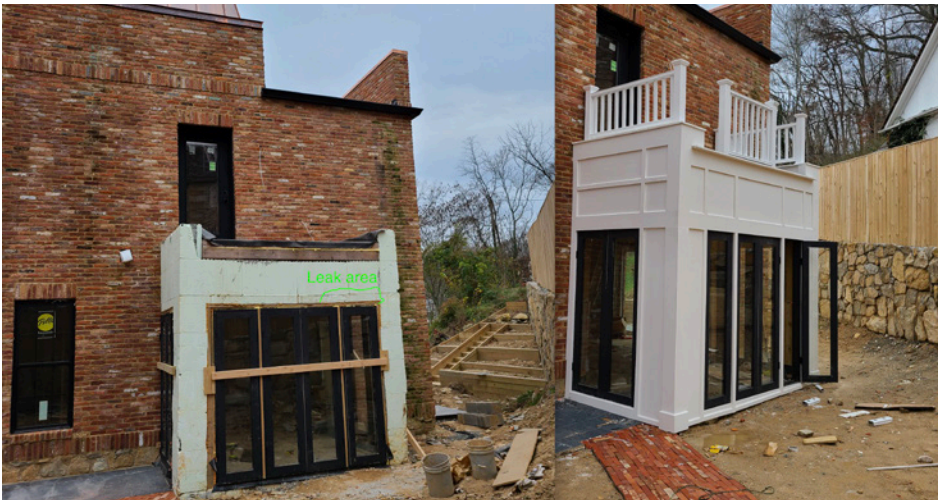
FIGURE 3. Doors and windows were installed without flashing.
