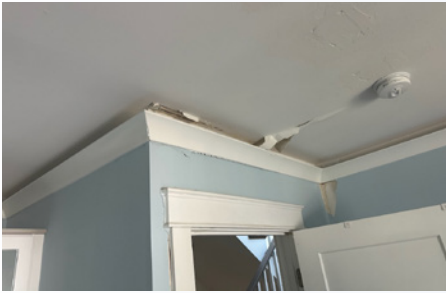
FIGURE 6. Water leaks appeared immediately.
