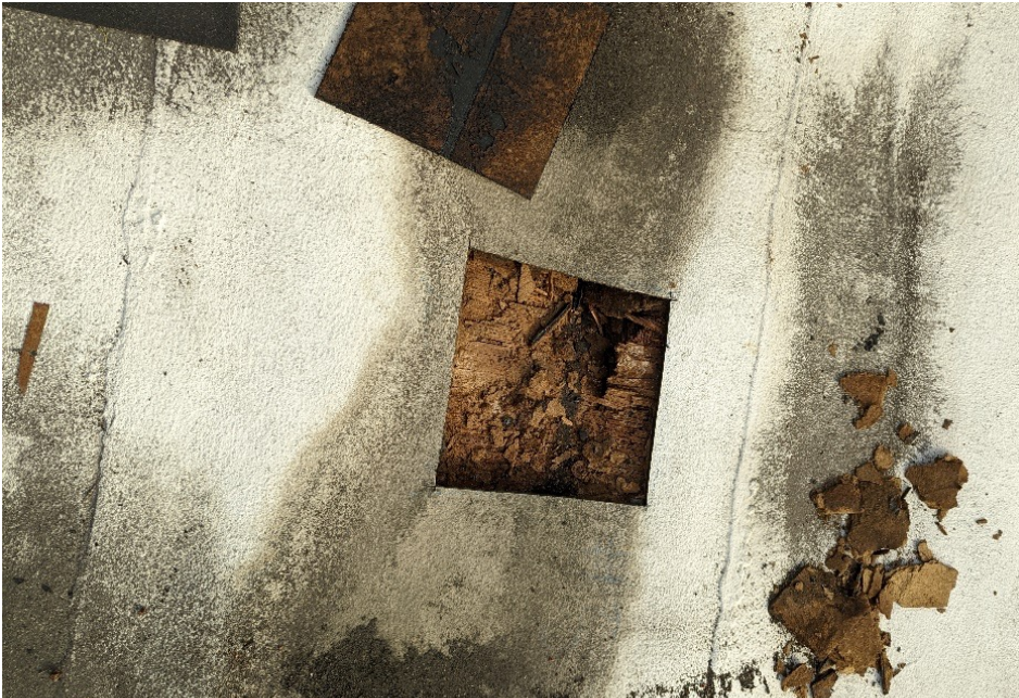
FIGURE 4. Example of condensation damage beneath a cool-roof membrane in Climate Zone 5.
