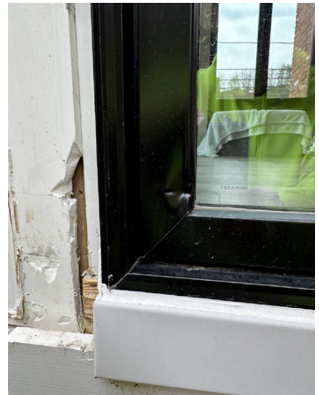
FIGURE 15. A window installer replaced the kitchen windows and doors, but did not add flashing and did not eliminate the water intrusion.
