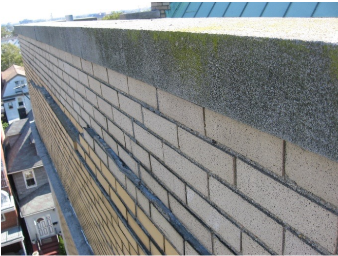
FIGURE 8. View of unsafe parapet masonry where it has shifted. Photo by author.
