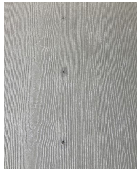
FIGURE 8. Water absorption at fastener penetrations.
