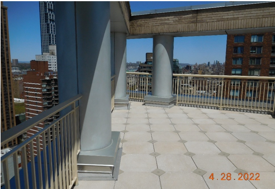
FIGURE 2. View of posted guardrail system with design that does not allow the passage of a 4 in. sphere. Photo by author.
