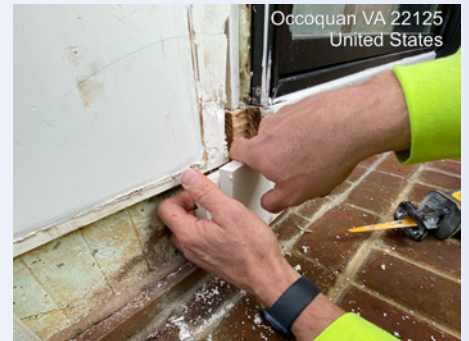
FIGURE 10. No flashing or waterproofing was present at the windows, as expected.
