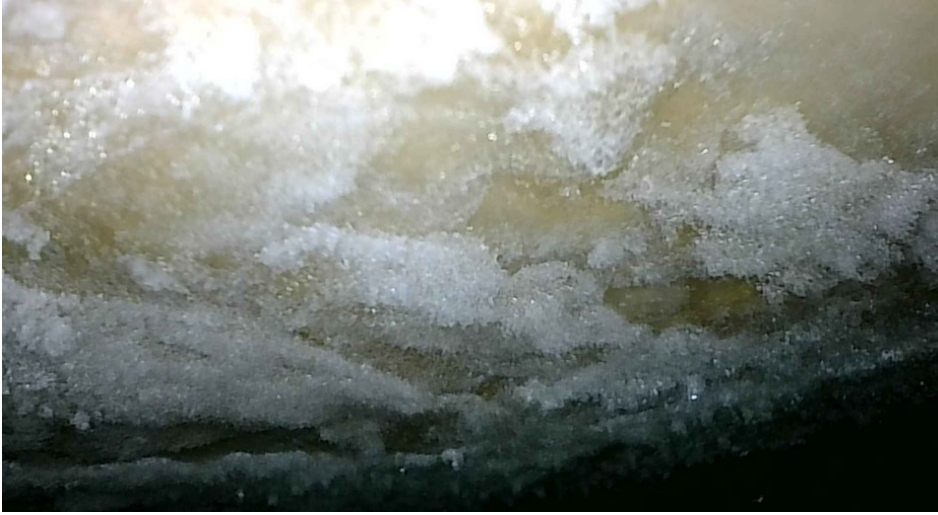
FIGURE 1. Frost buildup on the interior face of precast concrete.
