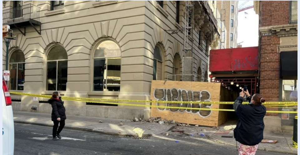
FIGURE 1. View of 2023 facade collapse debris in Philadelphia's Center City district. Image courtesy of 6ABC. 2
