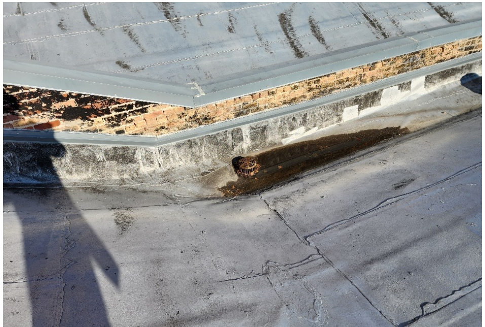
FIGURE 3. Example of a roof drain without a corresponding secondary (emergency overflow) drain or scupper.
