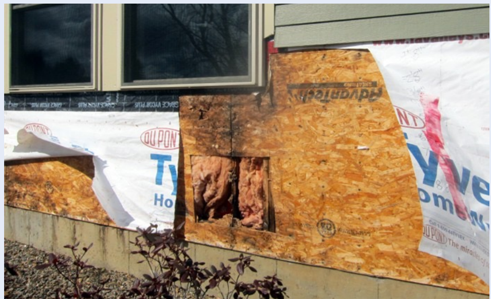
FIGURE 2. Natatorium wall failure.
