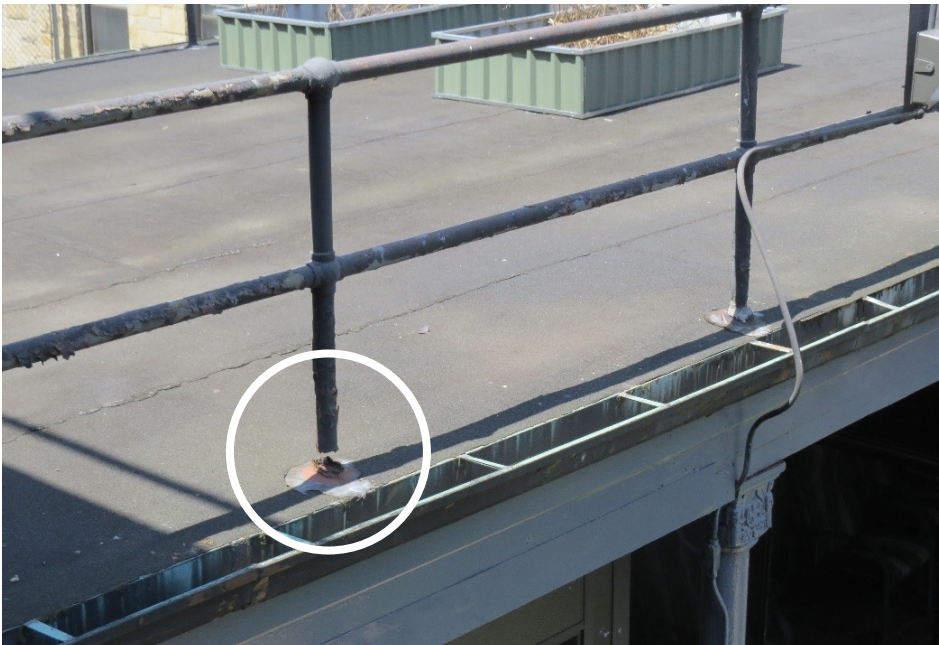
FIGURE 6. Posted guardrail completely corroded and post is left hanging. Photo by author.
