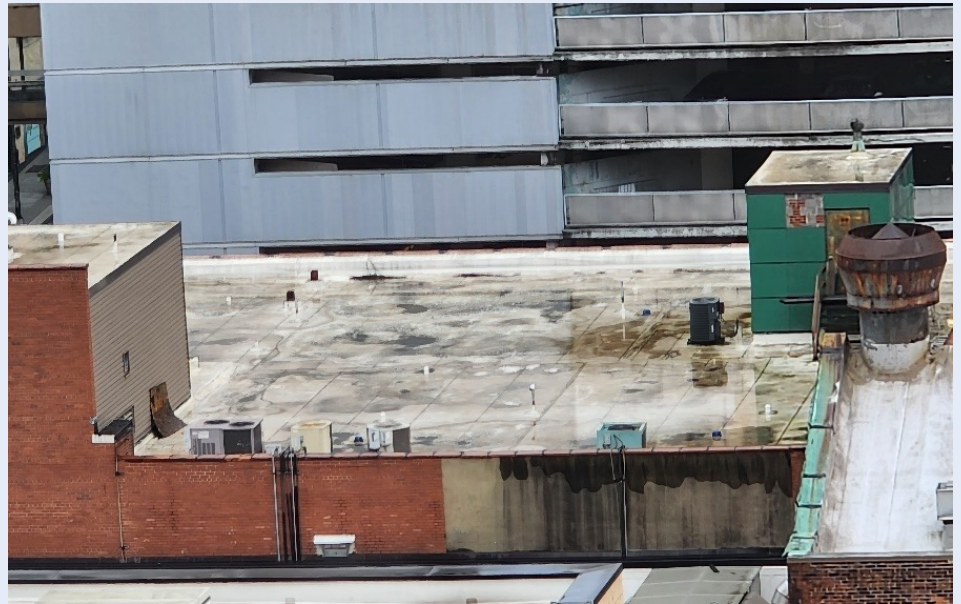
FIGURE 1. An underperforming roof.
