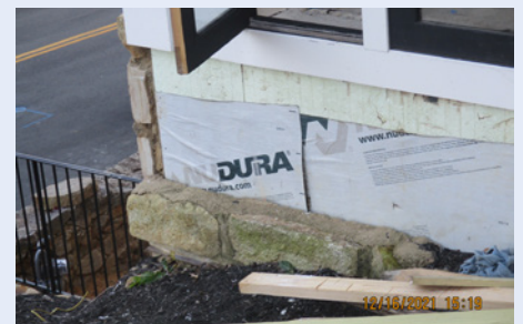
FIGURE 2. Waterproofing was applied without primer or termination bars.
