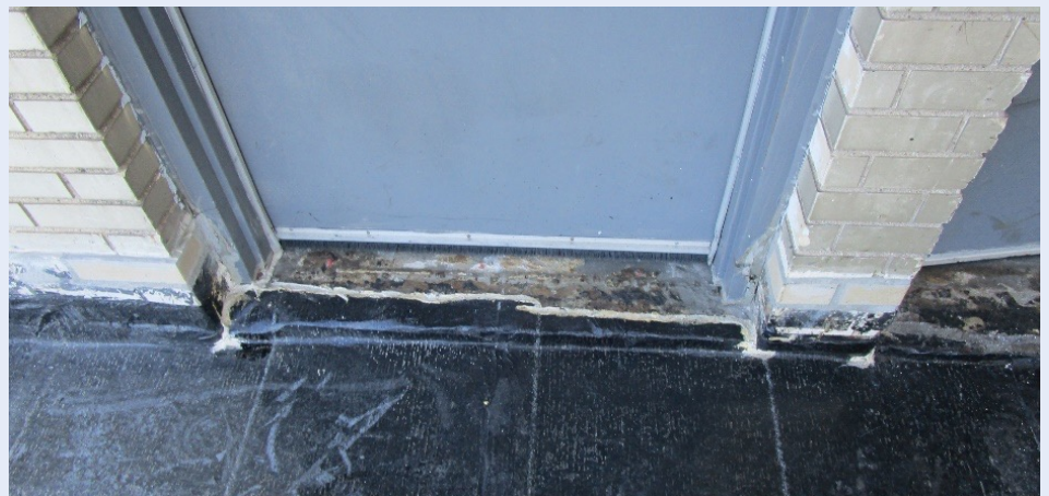
FIGURE 2. Example of a low door threshold height limiting adjacent roof system insulation thickness.
