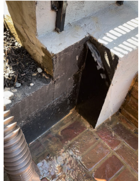
FIGURE 13. Photo of water “squirting” out of the retaining wall under hydrostatic pressure.
