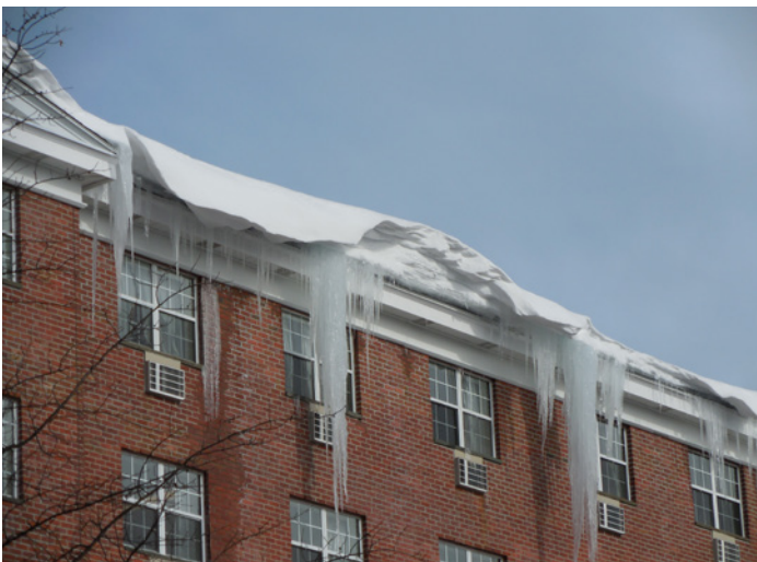
FIGURE 5. Ice dams and icicles resulting from insufficient ventilation.
