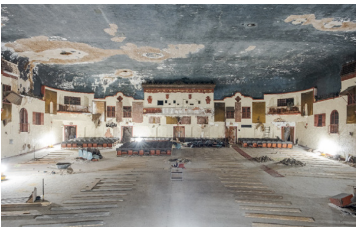
FIGURE 5. Interior view (from the stage) of the theater space showing the plaster conditions of the auditorium. Photo credit: Danielle Campbell.
