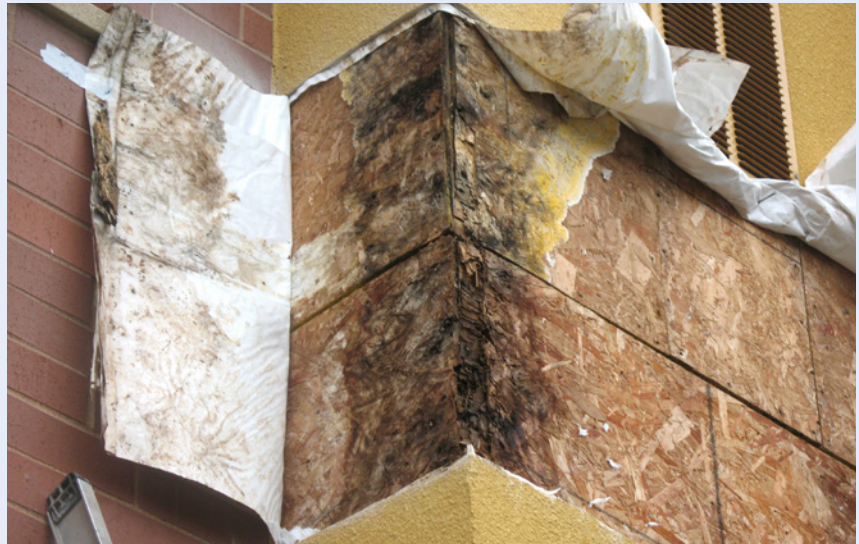
FIGURE 1. Material degradation due to cladding leaks and poor drainage.
