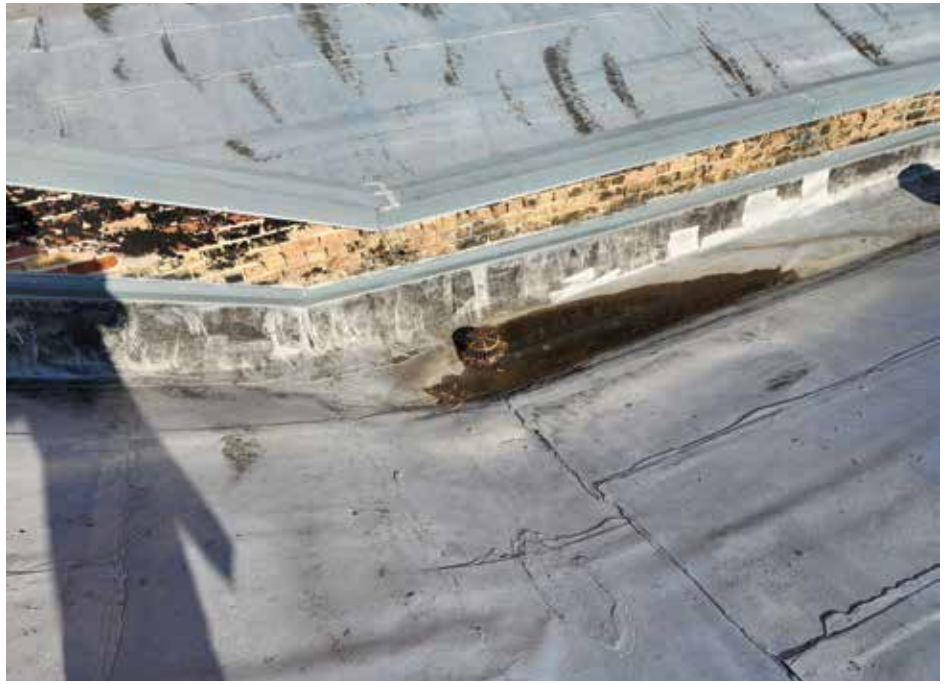
Figure 3. Example of a roof drain without a corresponding secondary (emergency overflow) drain or scupper. Courtesy of Klein & Hoffman.
