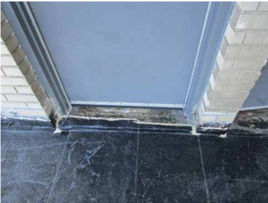
Figure 2. Example of a low door threshold height limiting adjacent roof system insulation thickness. Courtesy of Klein & Hoffman.
