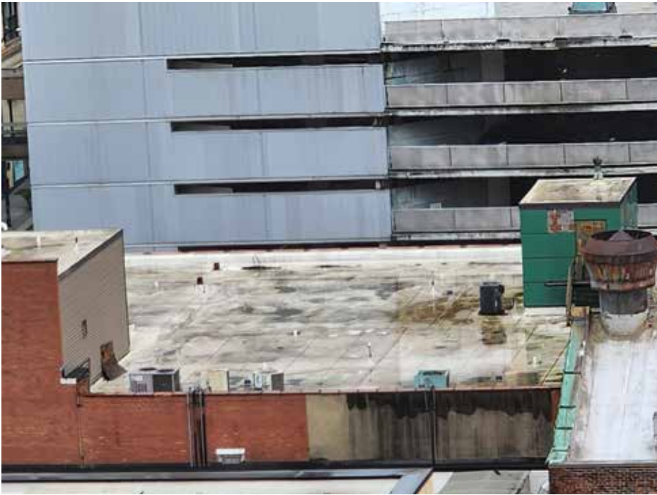
Figure 1. An underperforming roof. Courtesy of Klein & Hoffman.
