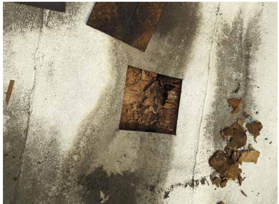
Figure 4. Example of condensation damage beneath a cool-roof membrane in Climate Zone 5. Courtesy of Klein & Hoffman.
