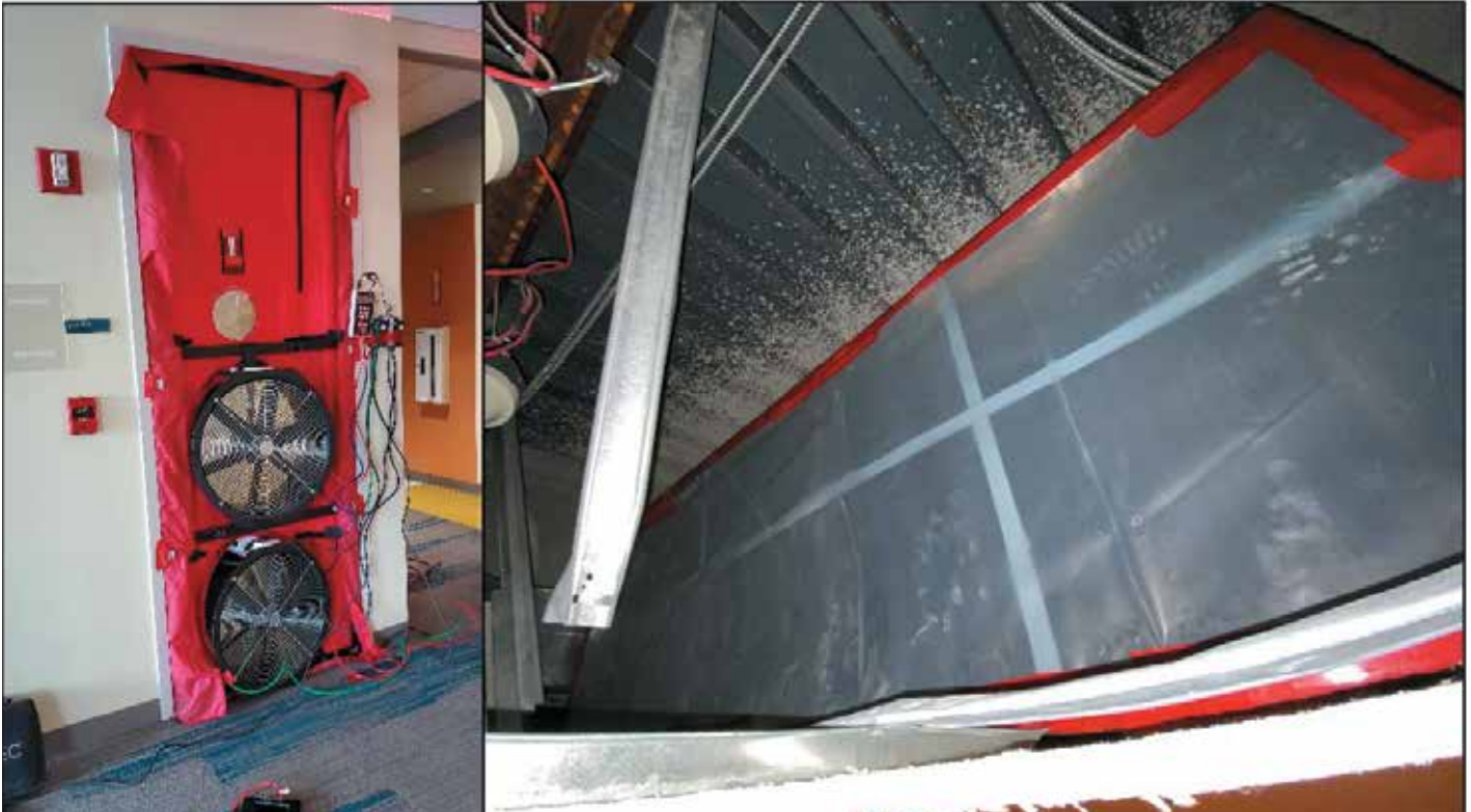
Figure 10. Whole-building airtightness testing issues: typical blower door fan setup at stairwell shaft (left) and large connecting plenums above suspended ceiling spanning multiple floors (right). Figure credit: Simpson Gumpertz & Heger Inc.
