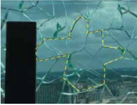
Figure 3. Close-up view of butterfly pattern of origin point within cracked glass.
