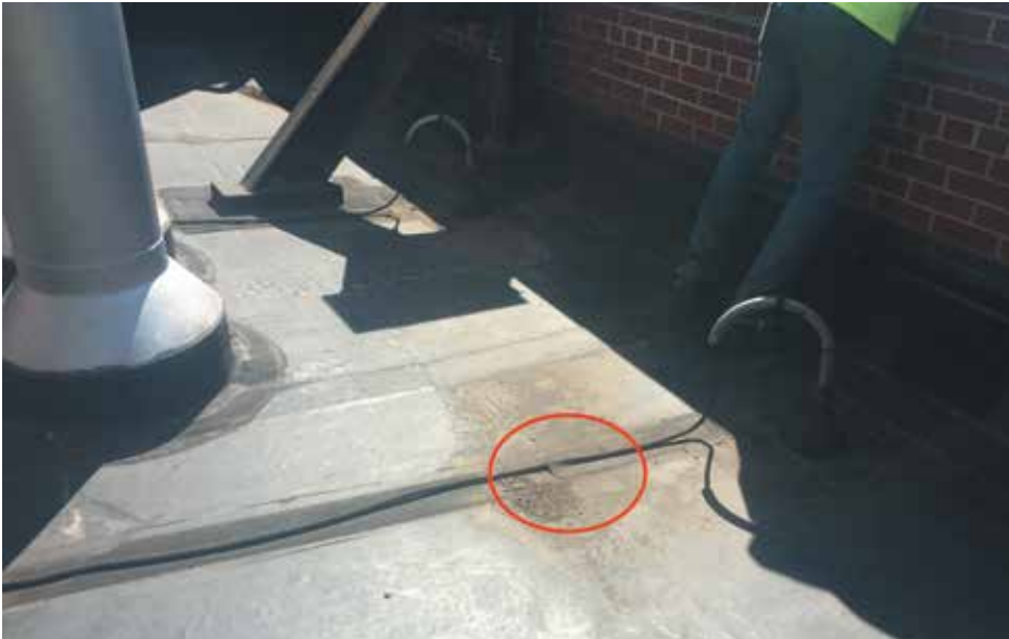
Figure 9. Inspection can identify inappropriate repairs or repairs that are necessary to ensure that a system remains functional. Here, a conductor has been repaired using a noncompliant method of securing the conductor to the roof.
