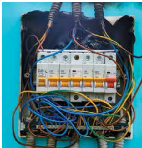
Figure 2. Damaged circuit board due to a lightning strike that caused a surge in the building.
