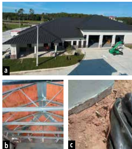
Figure 7. (a) An example of a community/critical facility, this Fort Myers fire station is located in a high-lightning-density zone. Early design coordination enabled a fully enclosed lightning protection system. (b) The installation team did not get the call to rough in the system before the top pour of the walls. Adjustments were made to conceal the system in the parapet wall. (c) Conductors through the wall “to ground,” which connect to the ground loop.
