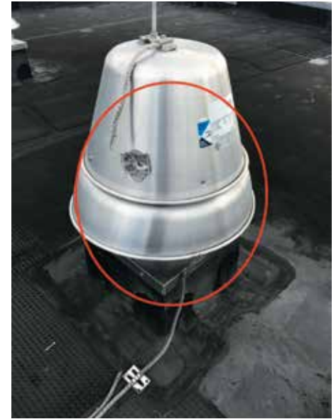
Figure 10. Rooftop equipment should be protected and monitored for damage due to possible other rooftop maintenance or issues.
