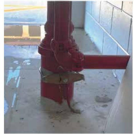
Figure 13. All conductive systems and metal bodies likely to become energized by lightning must be bonded to the lightning protection system to eliminate potential differences and reduce the risk of a side-flash.
