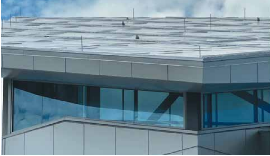
Figure 12. Close-up of the lightning protection system integrated into the roof of the US Air Force Academy's Visitor Center in Boulder, Colorado. Thorough assessment and coordination of trades are attributed to the design and sustainability of this structure.
