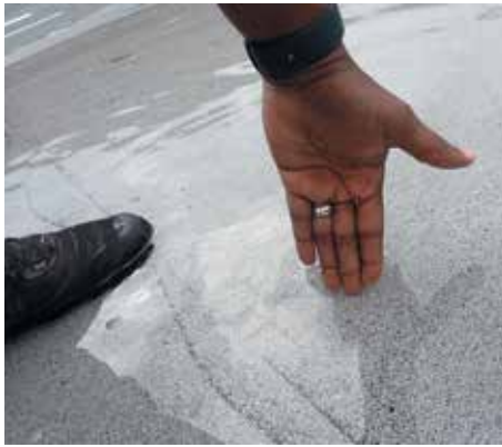
Figure 3. Field verification of ponding depth showing more than 1 in. (25.4 mm) of standing water between interior drains. The lack of adequate slope and missing secondary drainage pathways resulted in prolonged water retention following rainfall.
