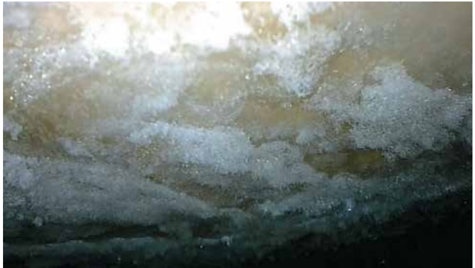
Figure 1. Frost buildup on the interior face of precast concrete.
