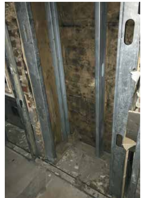
Figure 2. Organic growth at the interior face of the exterior sheathing within a neonatal intensive care unit space.
