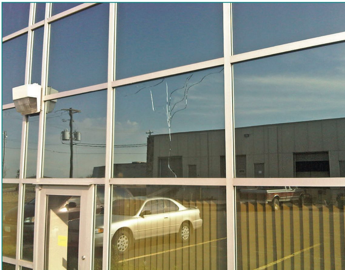
Figure 1 – Fractured heat-strengthened glass in a single-glazed curtainwall spandrel panel. The crack likely started at the bottom, extending into the center-of-glass region, before branching and continuing across the unit to the top.
