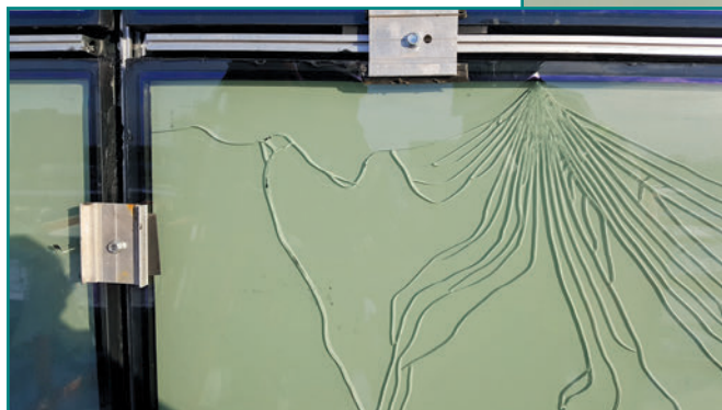
Figure 2 – Fractured heat-strengthened glass in an inboard pane of glass in an IGU of a curtainwall spandrel panel. The crack started at the upper left corner, to the right of the temporary restraint (dutchie) to the curtainwall frame behind, indicating a combination of thermal stress and mechanical stress contributed to breakage.
