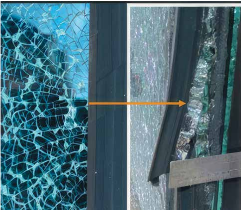
Figure 8. Close-up view of edge glass failure.
