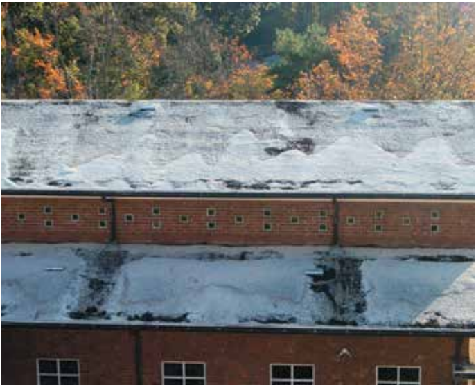
Figure 11. Downslope migration of bituminous flood coat and aggregate surfacing. The softening point of the bitumen was incompatible with the roof slope.
