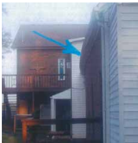
Figure 5. Outward bowing of walls of a church fellowship hall. Two large columns within had been removed, and the roof ridgeline slowly began sagging while walls responded by displacing outward at the top.
