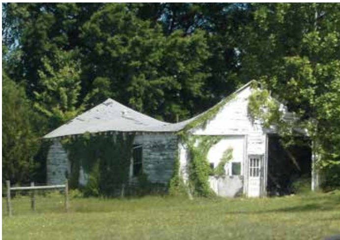
Figure 2. Extreme sagging of roof ridgeline and outward bowing of walls; this is a textbook example of long-term creep where lumber size and span relationships were substandard.
