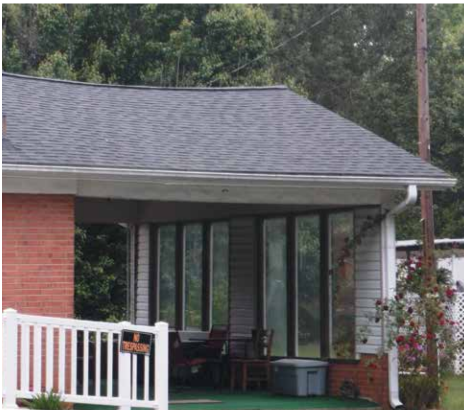
Figure 1. Sagging ridge beam in residential stick-built roof framing; this did not occur from a singular loading event.
