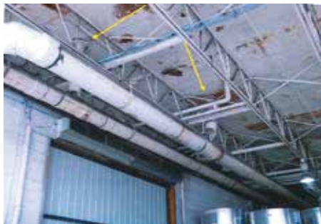
Figure 7. Internal drain lines running parallel to the direction of bar joists. This explains ponding only in a specific region on this roof; ponding had been present for decades.
