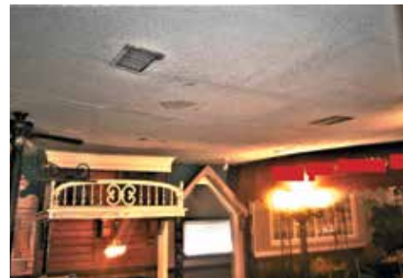
Figure 8. Severe ceiling sag in an occupied restaurant. Some instances of ceiling collapse are so abrupt and loud that witnesses have described an "explosion" in the attic.
