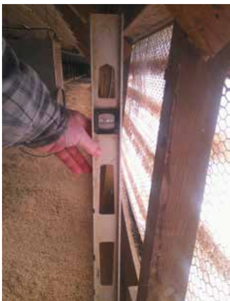
Figure 4. Another poultry confinement house (400 ft [122 m] long) experiencing extreme out-of-plumb leaning. Support posts and engineered roof trusses were 5 ft (1.5 m) on center, and ordinary shear diaphragm bracing was absent throughout.
