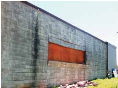
Figure 12. Unit masonry slumped vertically and eventually kicked out of plane. Decades in the making, it originated from a substandard connection to the backup plane.
