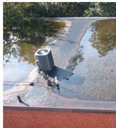
Figure 6. Severe deflection on a hollow-core concrete plank deck. High and dry region is that portion occurring above inside partition walls.
