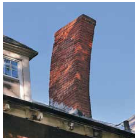
Figure 9. Radical curving of a brick masonry chimney, not from structural loading, but rather stemming from environmental influences over a long period.
