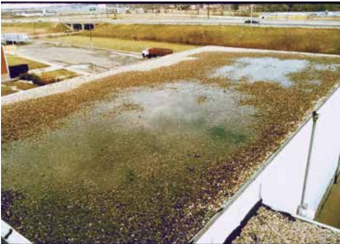
Figure 10. Older variety of structural insulated panel used for the walls and roof deck of a midwestern freezer facility. Severe deflection resulted from long-term ponding plus the mass of two roof layers (the outermost being stone ballasted). This behavior may be years in the making and well exemplifies creep.
