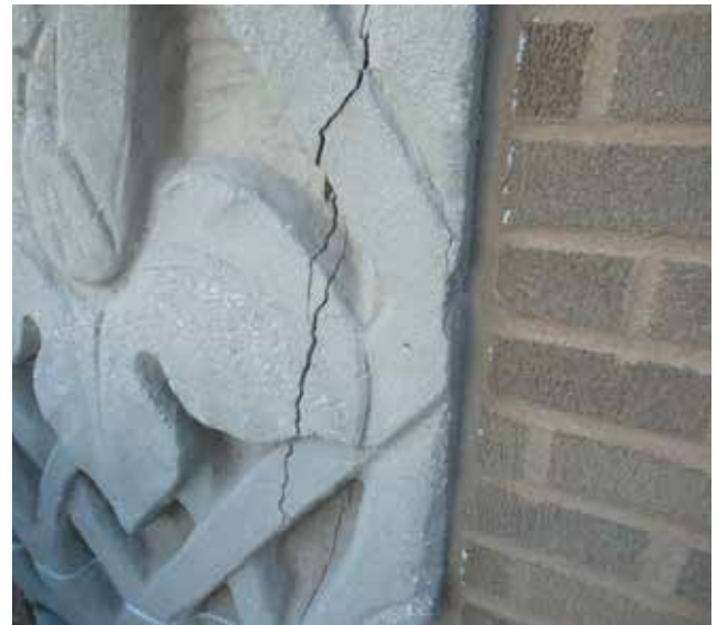
Figure 8. Close up view of cracked decorative stone at the Barclay-Vesey Building at 140 West Street. Photograph by Mike Lopez, November 21, 2022. Rimkus.
