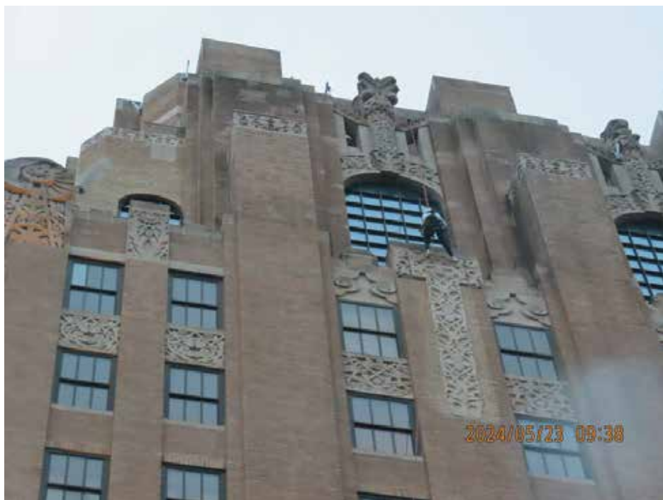
Figure 5. Inspector performing facade inspection via industrial rope access. Photograph by Mike Lopez, May 23, 2024. Rimkus.
