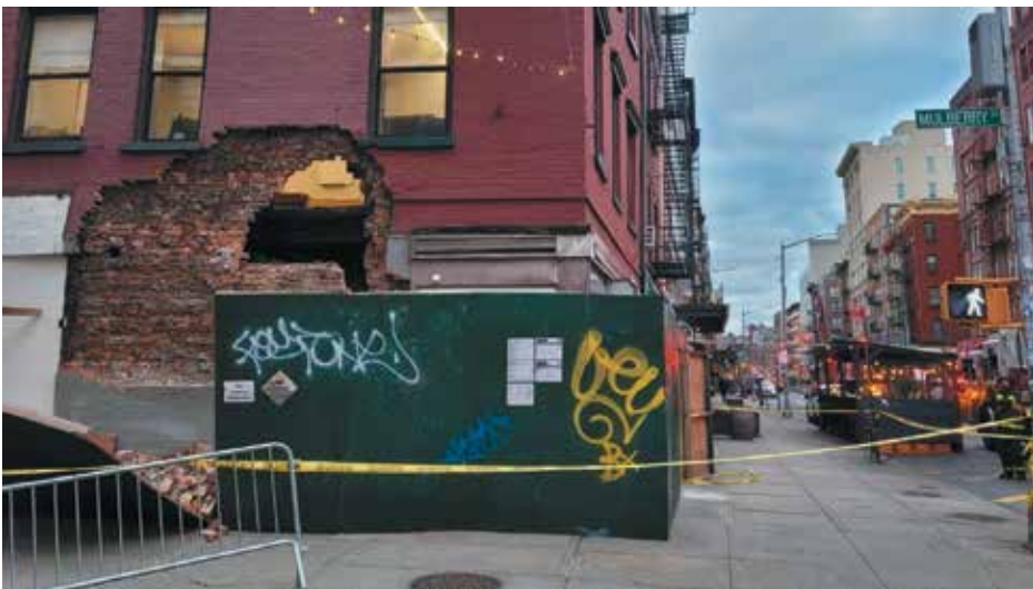
Figure 3. Facade collapse in New York City's Little Italy neighborhood. Image courtesy of The Structural Engineer. 7
