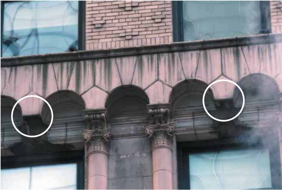
Figure 2. Close-up view of terra-cotta failure that led to fatality in New York City, 2019. Image courtesy of the New York Post. 4 Annotations by Mike Lopez.
