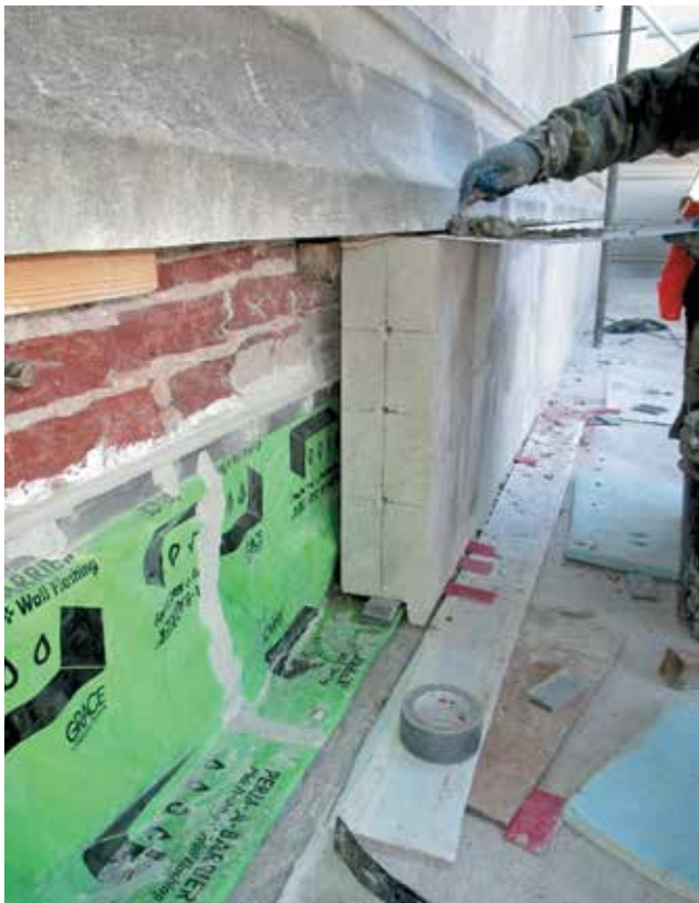
Figure 11. Installation of replacement stone at shelf angle location at 30th Street Station.
