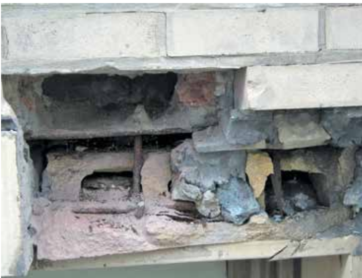
Figure 3. Distressed terra-cotta window head unit caused by corrosion of steel anchorages and support at Old Cook County Hospital as viewed during the 2011 Phase 1 assessment.
