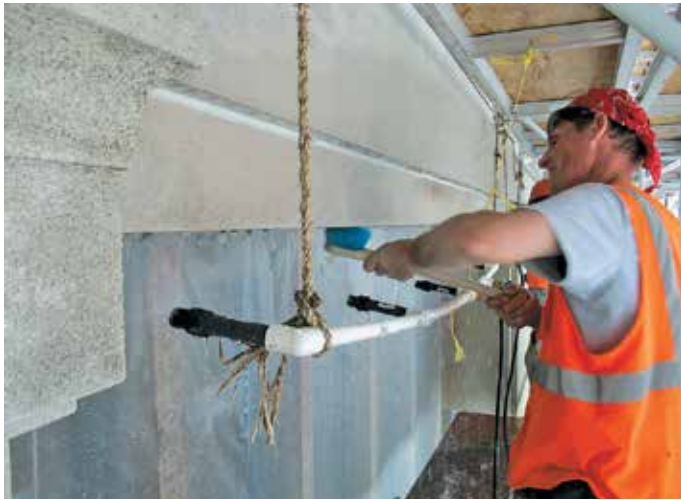
Figure 13. Water-misting cleaning at the limestone soffits at the main facades of 30th Street Station.
