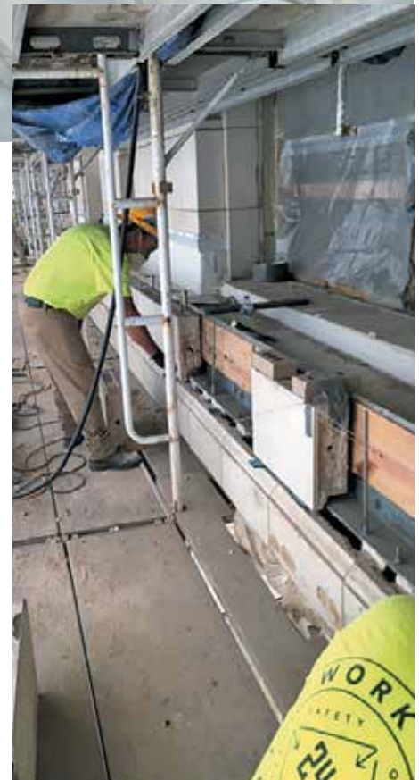
Figure 7. Reconstruction of the third-floor gutter and installation of terra-cotta units at the north, east, and west facades during rehabilitation of the Old Cook County Hospital in 2018–2019.
