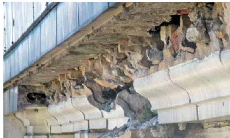
Figure 4. Distressed terra-cotta window on seventh-floor head units below a previously replaced cornice at Old Cook County Hospital, as viewed during the 2016 Phase 2 assessment. The distress was attributed to corrosion of steel anchorages associated with the poor detailing of the retrofit.
