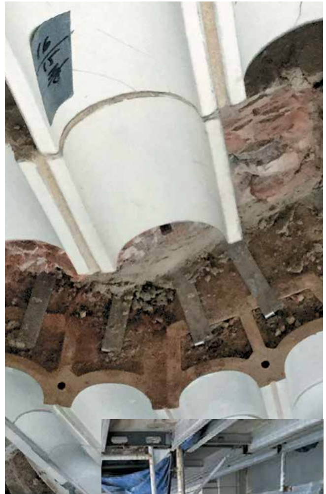
Figure 6. Installation of terra-cotta units at monumental columns at the north facade during rehabilitation of the Old Cook County Hospital in 2019.
