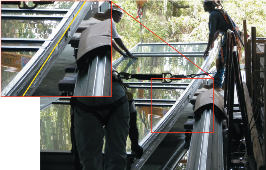
Figure 3. Excessive deflection of twin-span unitized curtainwall during erection.
