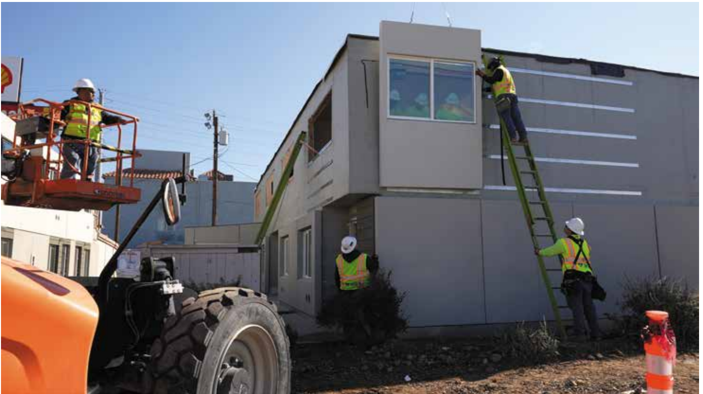
Figure 5. Prefabricated wall panels are raised with a crane and attached to the horizontal brackets on the building exterior.
