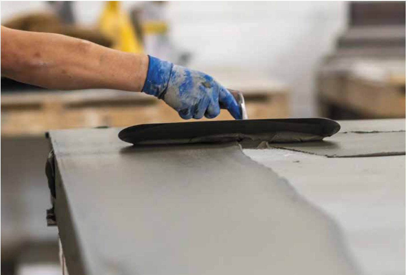
Figure 4. A worker applies finishing material to an exterior wall panel in a factory.
