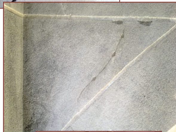
Figure 27. Stone crack after grout injection.
