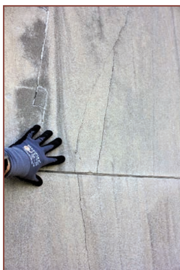
Figure 6. Cracks that will allow water to enter the stone.
