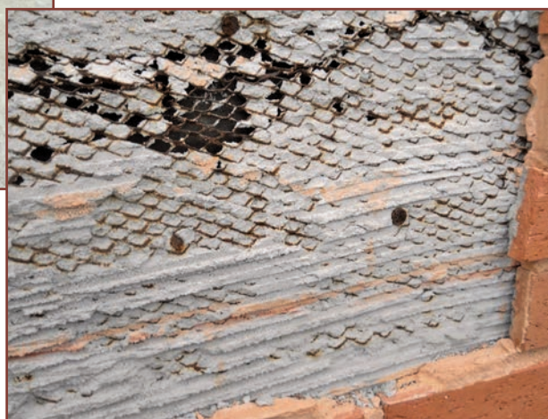
Figure 4. Poorly embedded metallic lath resulted in corrosion, pop-offs, and compromised anchorage.
