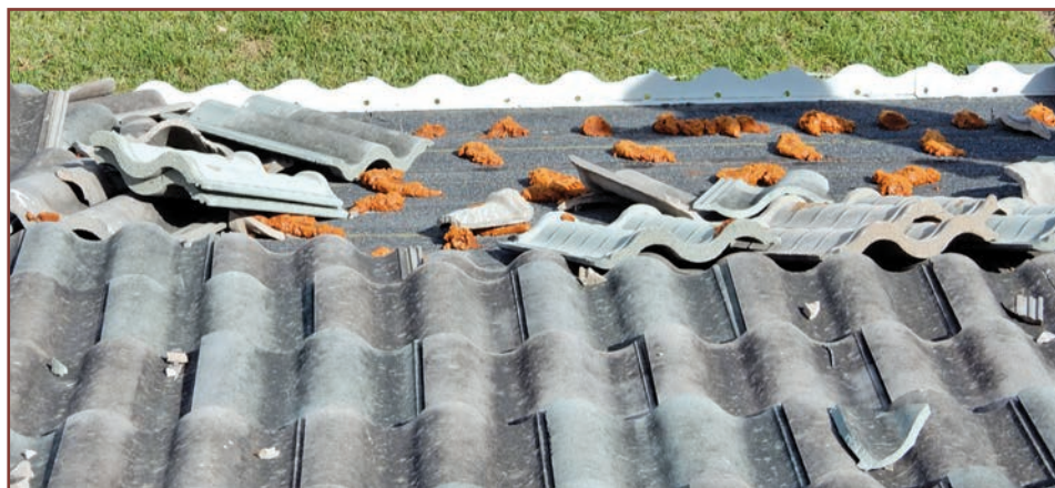
Figure 7. Hurricane Irma: Winds 100 to 110 mph. Inadequate adhesion.
