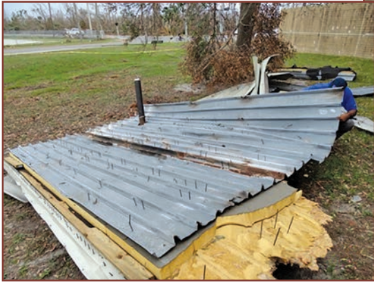
Figure 10. Metal panels where the perimeter was not fastened to the edge nailer.
