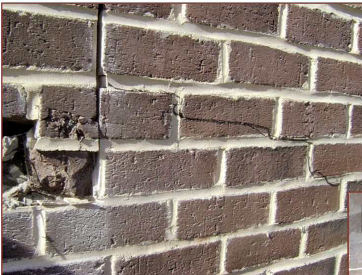
Figure 6. Cracking noted in manufactured stone veneer in area that correlated with dissimilar backup materials.
