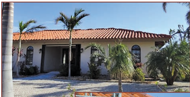
Figure 5. Hurricane Irma: 110 to 120 mph winds. Typical tile damage. Foam adhesive; damage limited to tiles missing from ridge.
