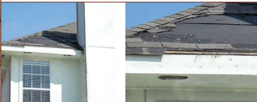
Figure 17. Typical damage to a roof installed using the racking method.
