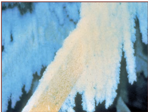
Figure 7. Frost in attic.
