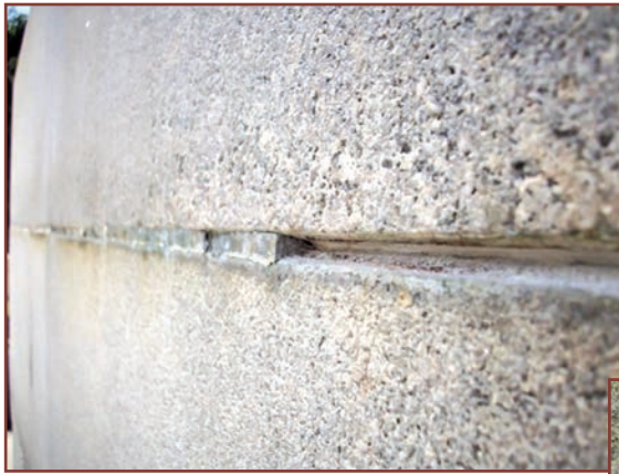
Figure 34. Failed joint repointing and widened joint.
