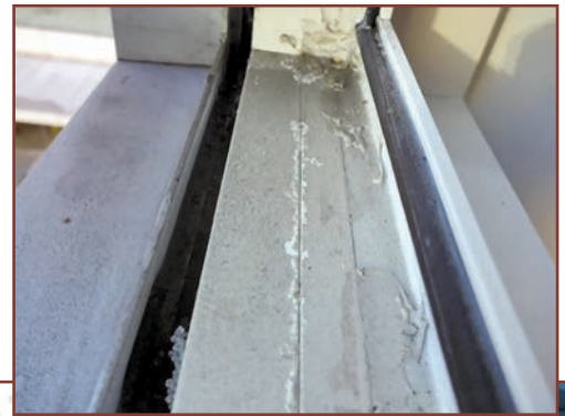
Figure 8. Polyvinylidene fluoride coating failure: Corrosion at aluminum window wall frame.
