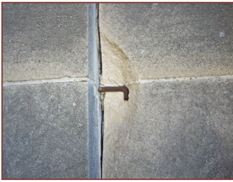
Figure 15. Spall caused by corrosion of a stone anchor.
