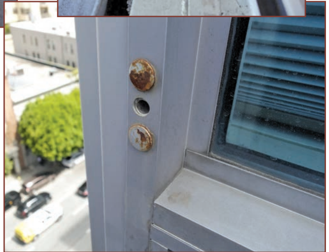
Figure 9. Polyvinylidene fluoride coating failure: Corrosion at window wall tie-back ports.
