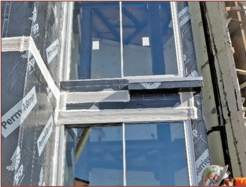
Figure 12. Failed original joint installation.
