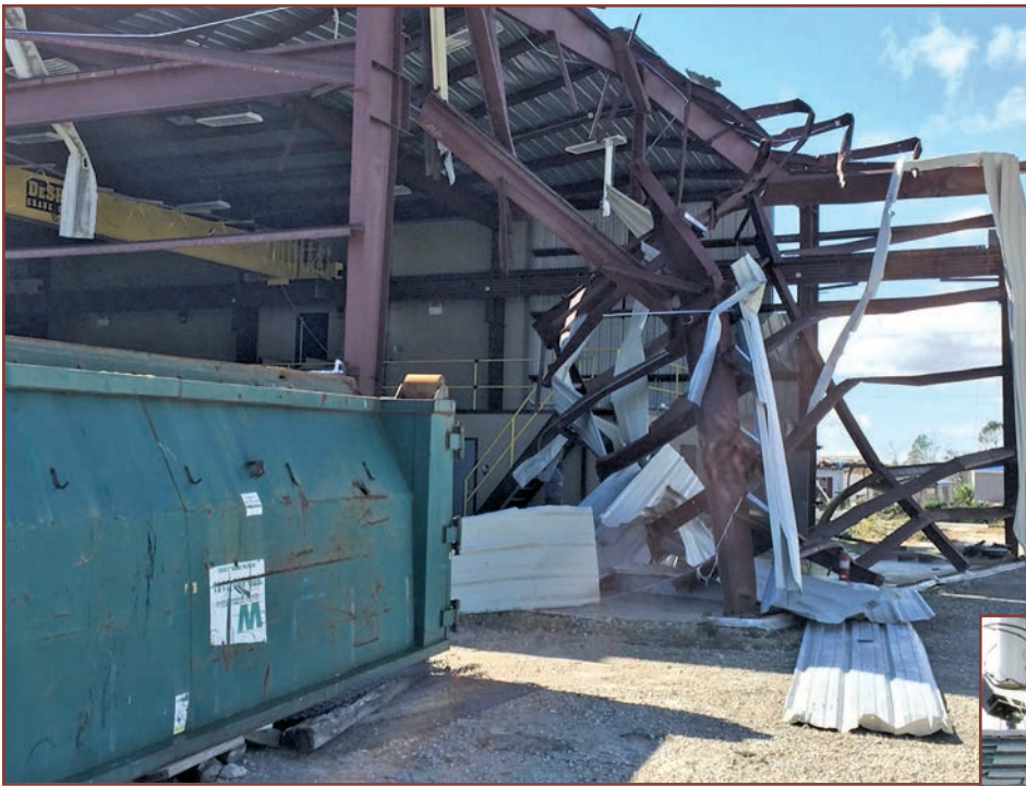
Figure 13. Hurricane Michael: 140 mph winds. This open metal building had cladding and roof loss. Many of the connections were corroded.
