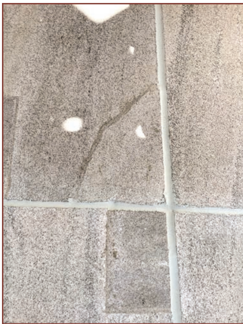
Figure 24. Reattached stone fragment.
