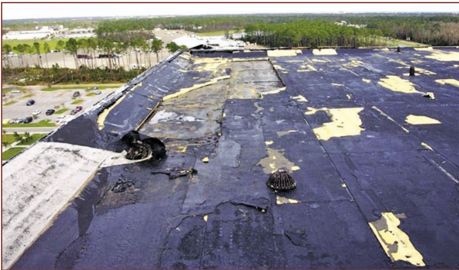
Figure 2. Damage to the Pensacola Naval Hospital in Florida from Hurricane Ivan.
