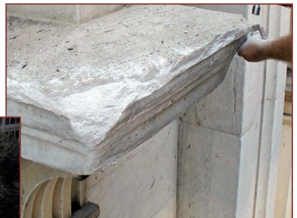
Figure 13. Weakening of a marble cornice due to hysteresis.
