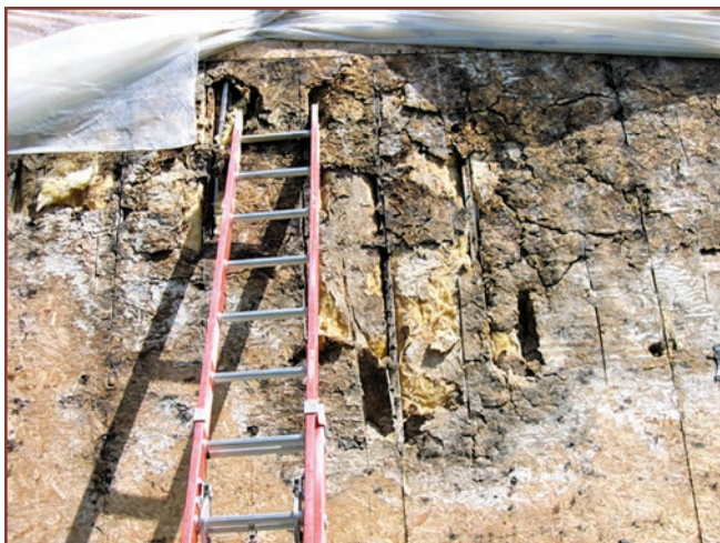
Figure 9. Rotten, five-year-old walls.
