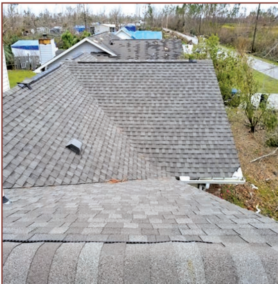
Figure 16. Hurricane Michael. Relatively new roof 2018 with some ridge and corner damage, older roofs in background with damage.
