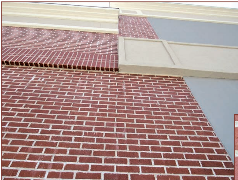
Figure 8. Large area of manufactured stone veneer without any control joints.
