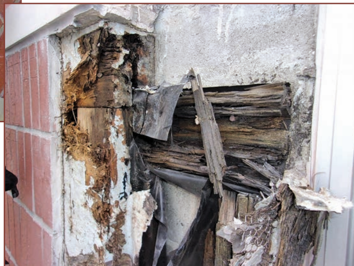
Figure 2. Poorly integrated/installed water-resistant barrier and flashing behind manufactured stone veneer allowed for significant water intrusion, damage, and swollen substrates.
