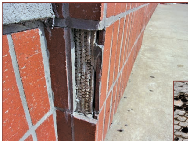
Figure 3. Poorly embedded lath and associated corrosion.
