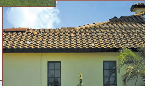
Figure 2. Hurricane Charley: 130 mph and greater winds. Typical ridge damage with downslope breakage due to tile debris. Mortar adhesive.
