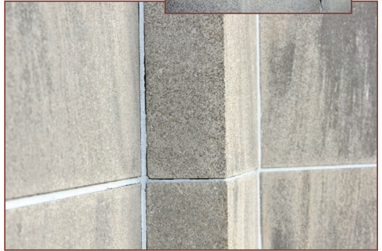
Figure 12. Failed sealant allows water to reach stone anchors and ultimately the building interior.
