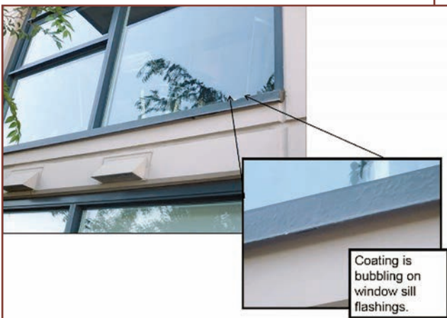
Figure 10. Polyvinylidene fluoride coating failure: Significant corrosion at window flashings.
