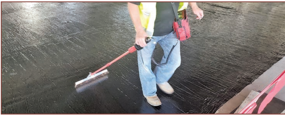
Figure 2. Electronic leak detection—high voltage.
