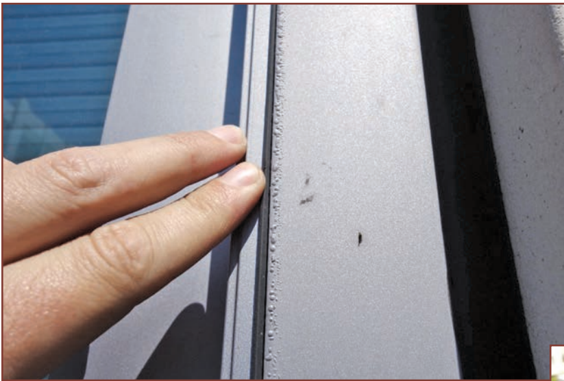
Figure 7. Polyvinylidene fluoride coating failure: Corrosion at aluminum window wall frame.
