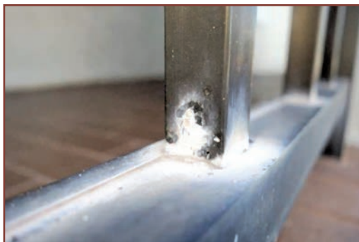
Figure 1. Corrosion (white oxide layer) on anodized aluminum guardrail.
