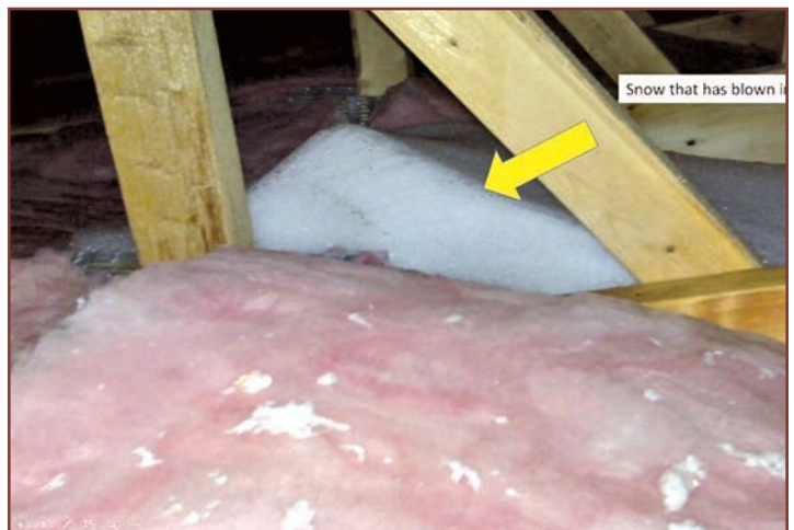
Figure 3. Snow in attic.
