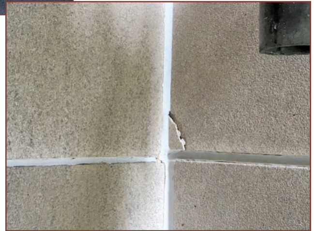
Figure 19. Small incipient spall near joints that will contribute to water infiltration if left unrepaired.
