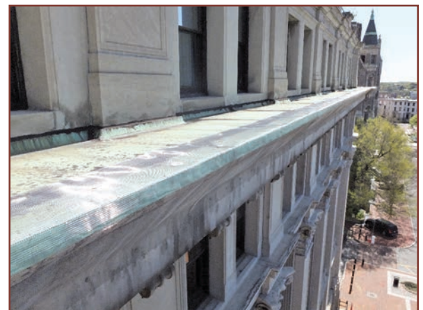
Figure 17. A limestone cornice is vulnerable to weathering, but partially shields the limestone facade below.
