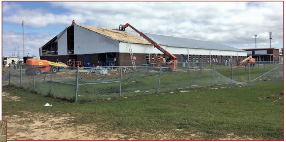
Figure 11. Hurricane Michael: 140 mph winds. The brick wall was inadequately supported and collapsed, allowing this building to be overpressurized. The roof damage stopped at a floor-to-roof separator.
