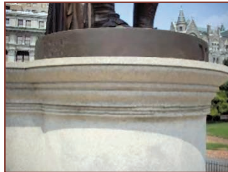
Figure 16. Minor chipping that would require a complex dutchman profile to repair.
