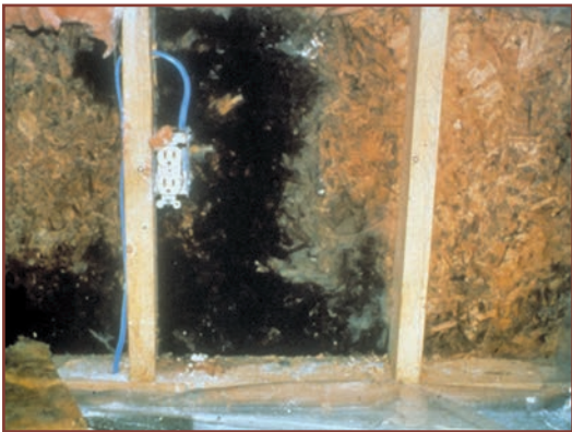
Figure 8. Mold on sheathing.
