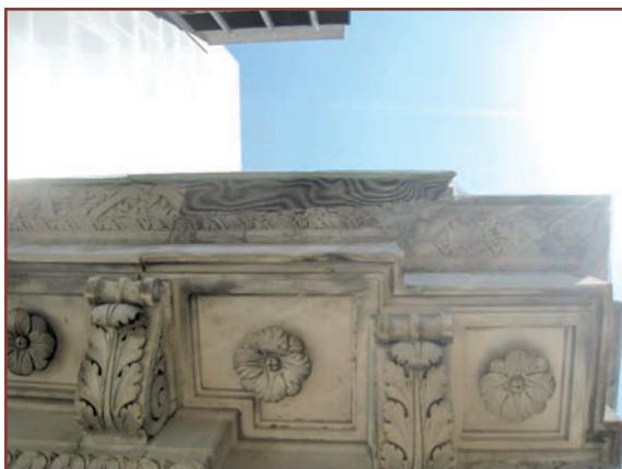
Figure 5. Large spall failure at a limestone cornice.
