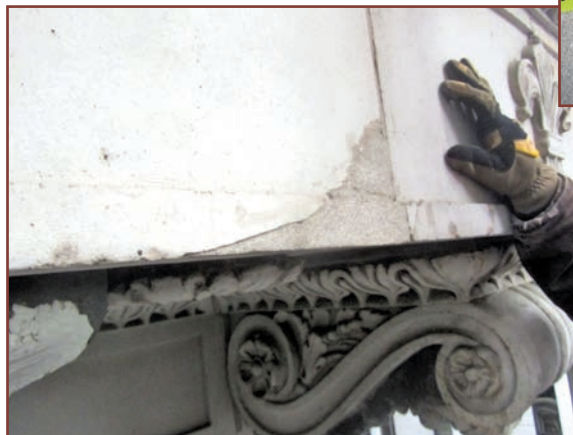
Figure 37. Poorly installed and placed patch.
