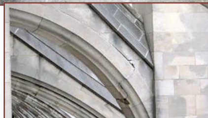
Figure 28. A critically damaged load-carrying stone element.
