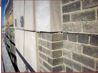
Figure 10. Displaced stone facade unit.
