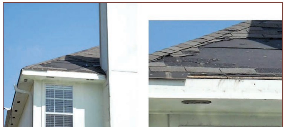
Figure 15. Hurricane Michael. Corner of roof with damage. Excessive overhang of starter course. First course not sealed.
