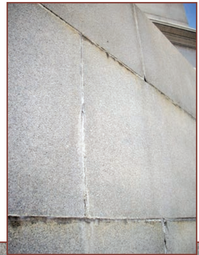
Figure 11. Failed joint mortar has led to water infiltration and efflorescence.
