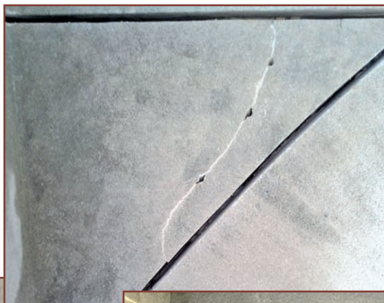
Figure 26. Stone crack prior to grout injection.
