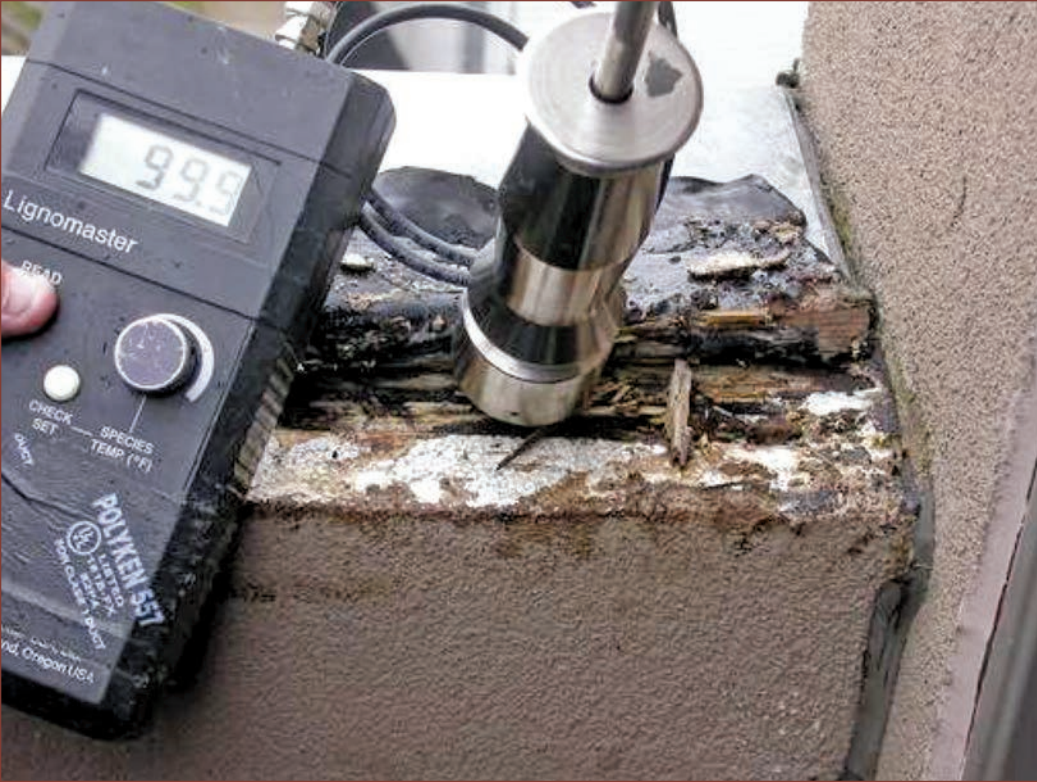
Figure 3. Deteriorated and wet wood blocking at a parapet-to-wall condition.
