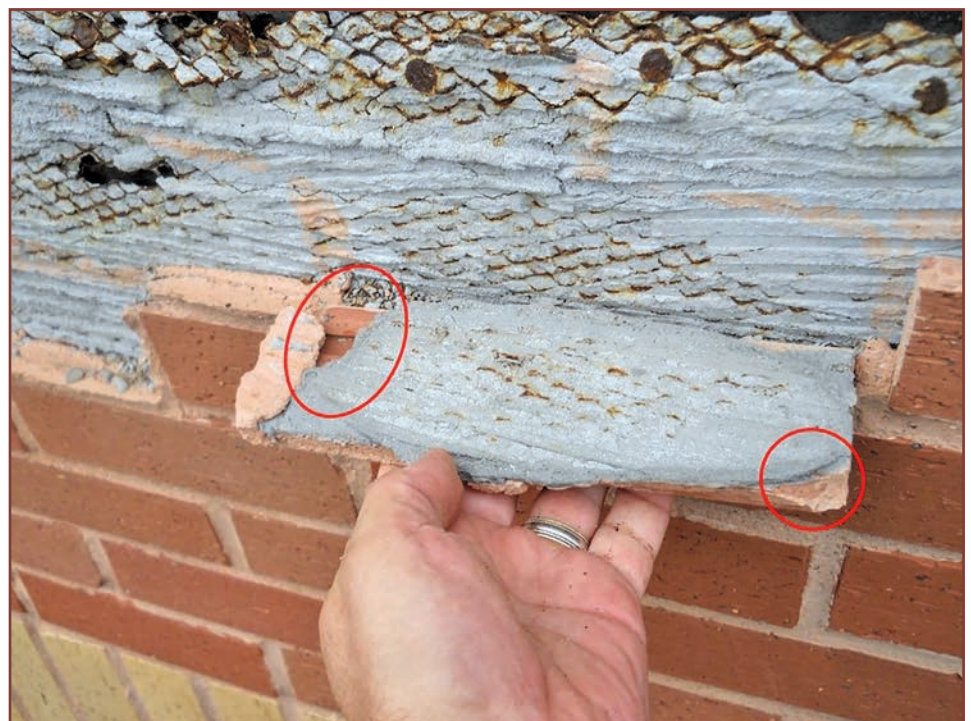
Figure 10. Incomplete setting bed resulted in voids/pockets behind the adhered brick veneer.
