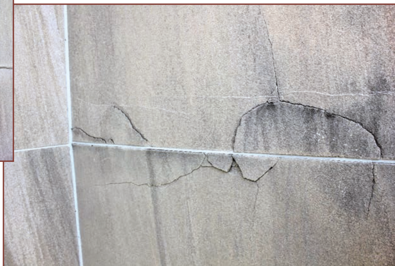
Figure 7. Incipient spalls located along a stone joint.
