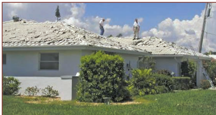
Figure 1. Hurricane Charley: Likely 140 mph winds. Typical damage in this older subdivision. Tiles using mortar as the adhesive.
