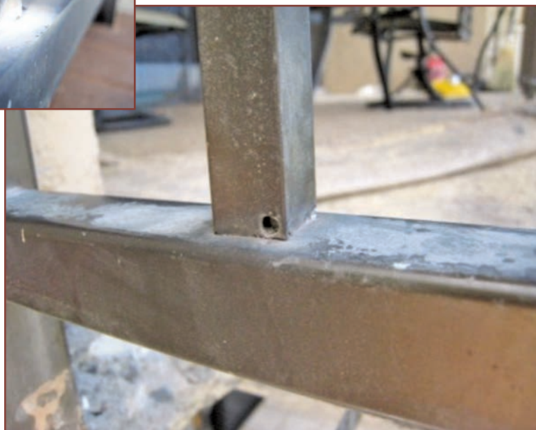
Figure 2. Galvanic corrosion on anodized aluminum guardrail.
