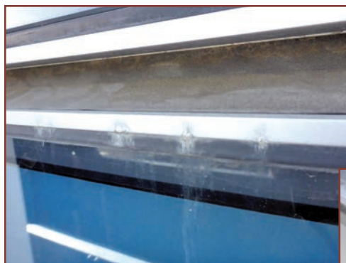
Figure 5. Polyvinylidene fluoride coating failure: Corrosion at aluminum curtain wall frame.
