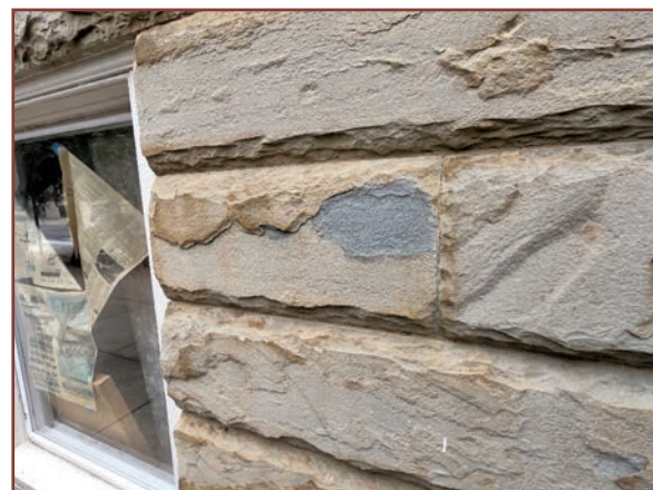
Figure 8. Failure of "face bedded" stone facade units along the bedding planes.
