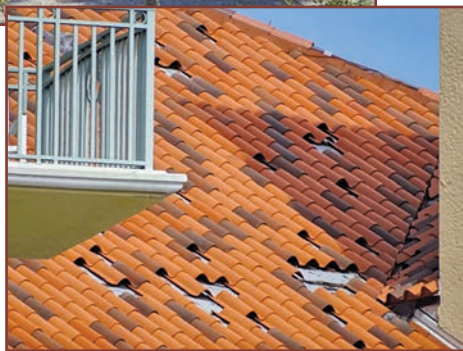
Figure 6. Hurricane Irma: 100 to 110 mph winds. Tiles installed with two nails; displaced ridge tiles damaged downslope tiles.
