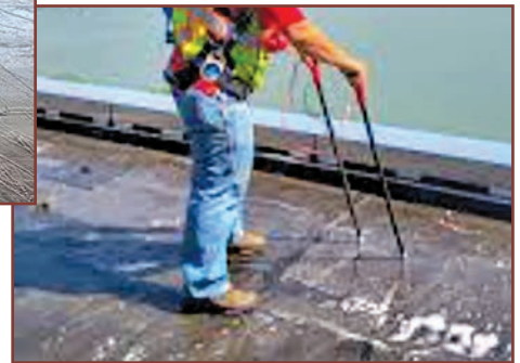
Figure 6. Low-voltage electronic leak detection.
