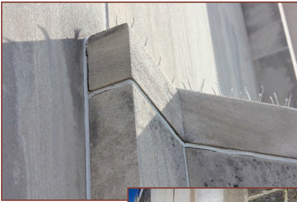
Figure 9. Displaced stone coping unit.
