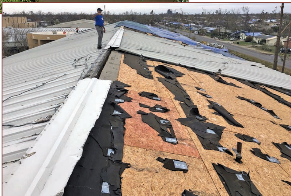
Figure 9. Hurricane Michael: 140 mph winds. This metal-panel roof was blown off. One of the weak links was the edge fasteners totally missing the edge nailer. This roof also had significant internal pressurization from failed soffits.
