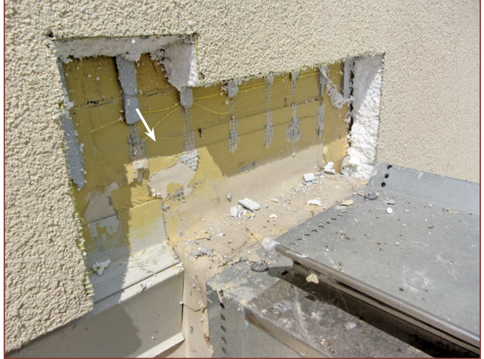
Figure 6. Some integration of the roofing membrane with the air/moisture barrier behind the exterior insulation and finish systems drainage system. However, no transition flashing was provided to integrate the roofing membrane termination to the air and moisture control layer (arrow).
