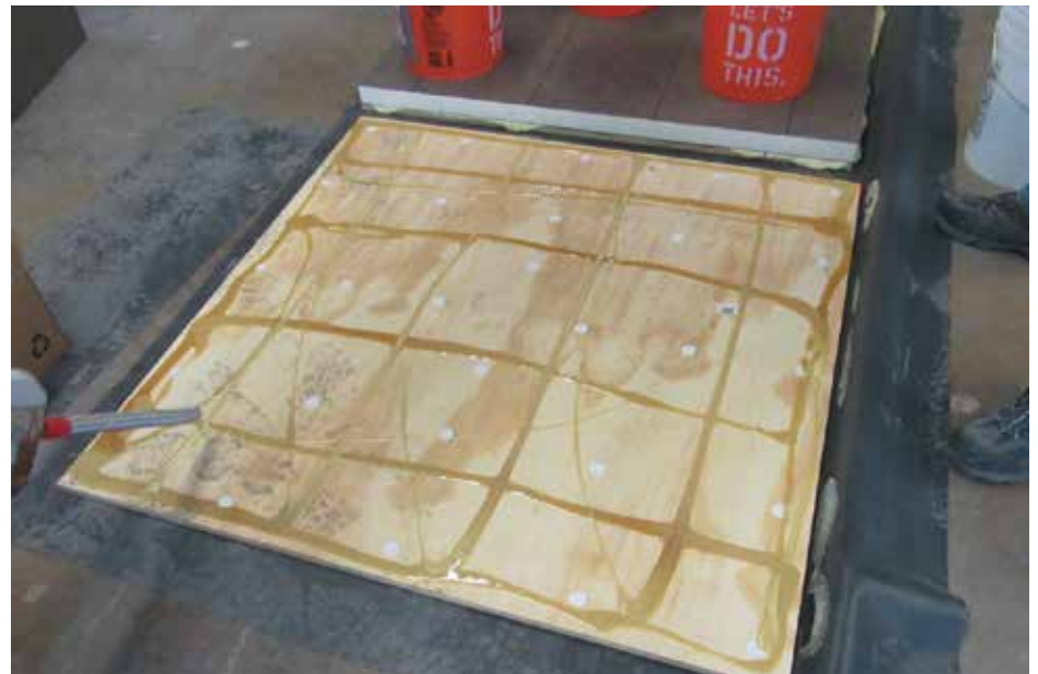
Figure 2. Grid of low-rise foam adhesive being applied to plywood panels to achieve an approximate 6 in. grid onto which one of the insulation boards would be placed.
