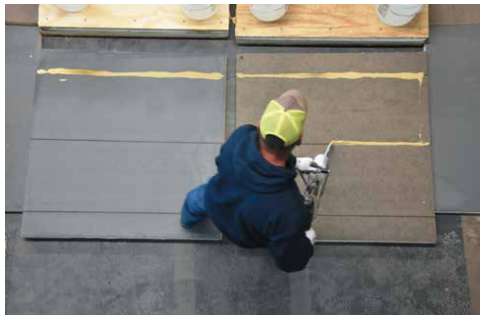
Figure 3. Typical low-rise foam adhesive bead width being applied to two separate insulation boards with 18 in. ribbon spacing lines.
