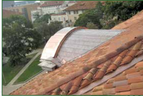
Carothers Dorm showing the copper on the barrel dormer, tile, and a copper valley flashing.
