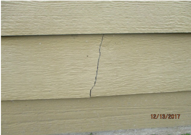
Figure 9 – Close-up view of crack in fiber-cement siding.
