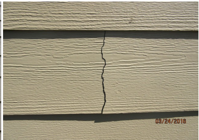
Figure 2 – Close-up view of crack in fiber-cement siding.
