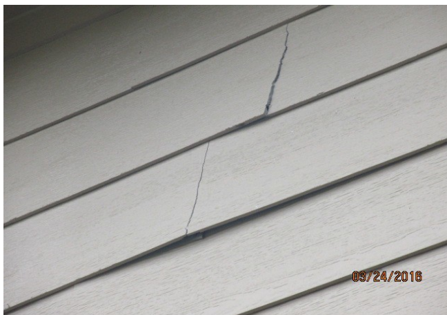
Figure 3 – Cracks and “warping” in fiber-cement siding.
