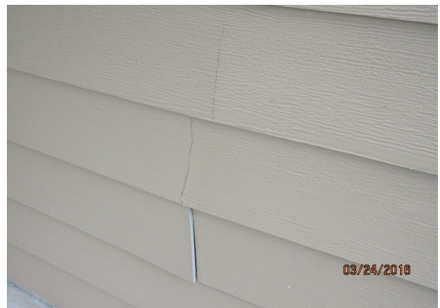
Figure 4 – Cracks and “warping” (open joint) in fiber-cement siding.
