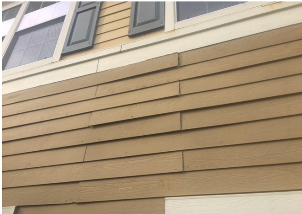
Figure 7 – Warped fiber-cement siding panels and opened butt joints between panels.
