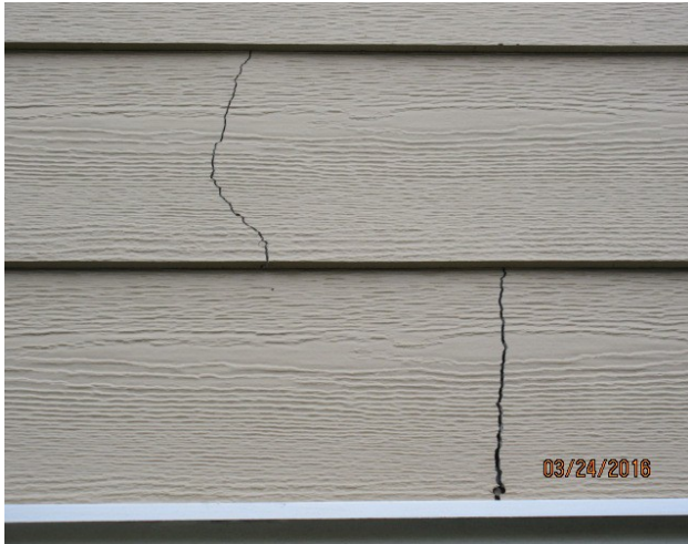
Figure 5 – Close-up view of cracks in fiber-cement siding.
