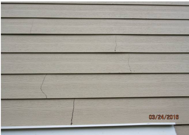
Figure 1 – Cracks in fiber-cement siding.
