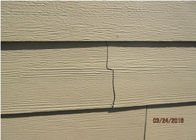
Figure 6 – Close-up view of cracks in fiber-cement siding.
