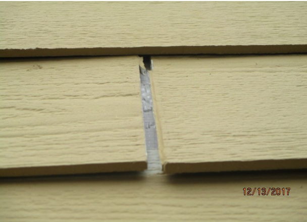
Figure 10 – Close-up view of open butt joint in fiber-cement siding.
