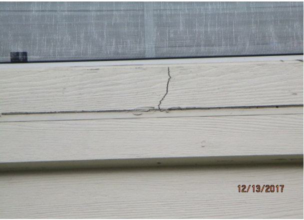
Figure 8 – Crack in fiber-cement trim.
